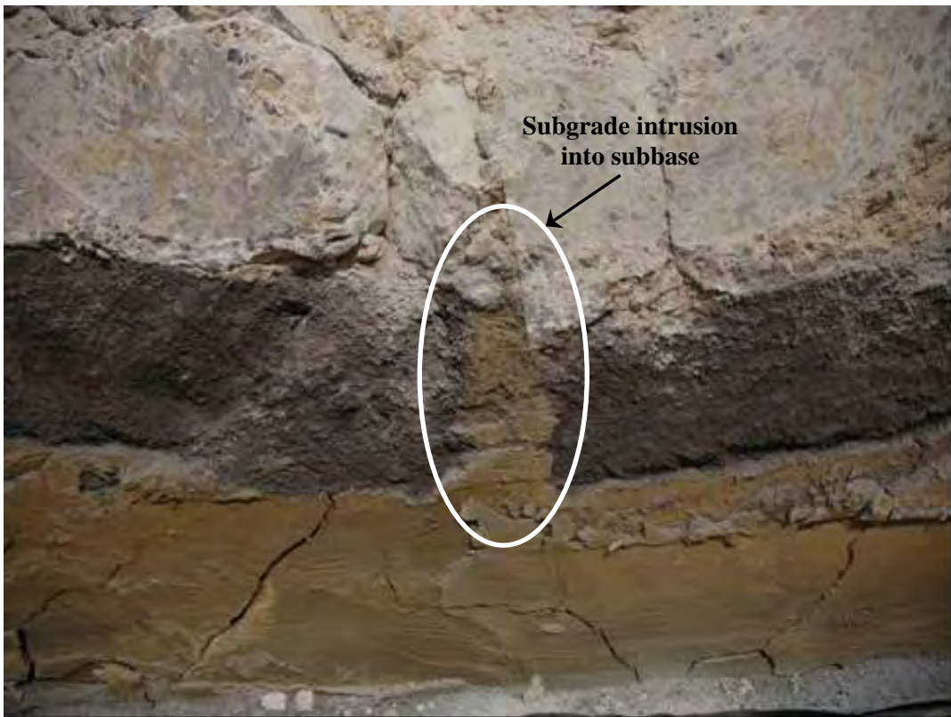
Figure 27. Subgrade Intrusion Into Subbase (MRC-E)
