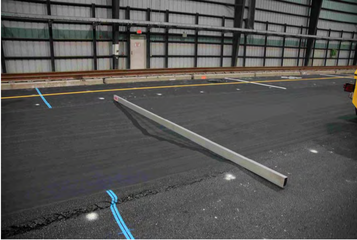
Figure 18. Pavement Failure in the East End of Rubblized Test Item MRC
