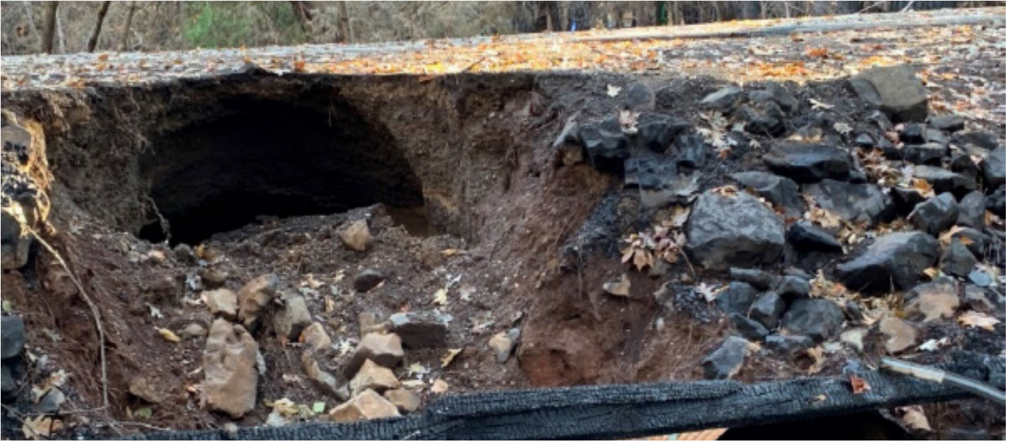
Figure 5. Photo. Collapsed culvert after Camp Fire (Mattox 2020).
