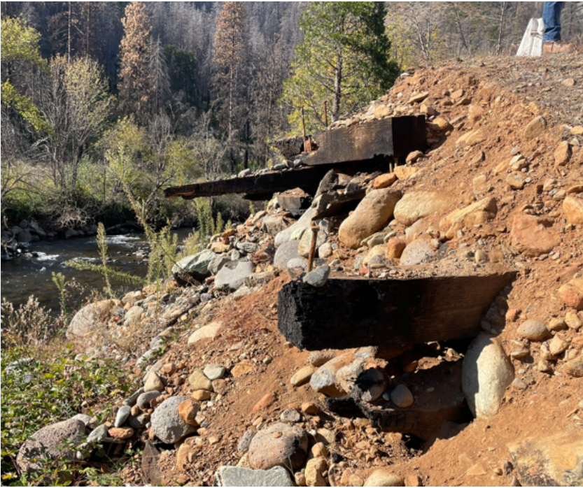
A. Timber substructure elements with signs of severe fire damage.
