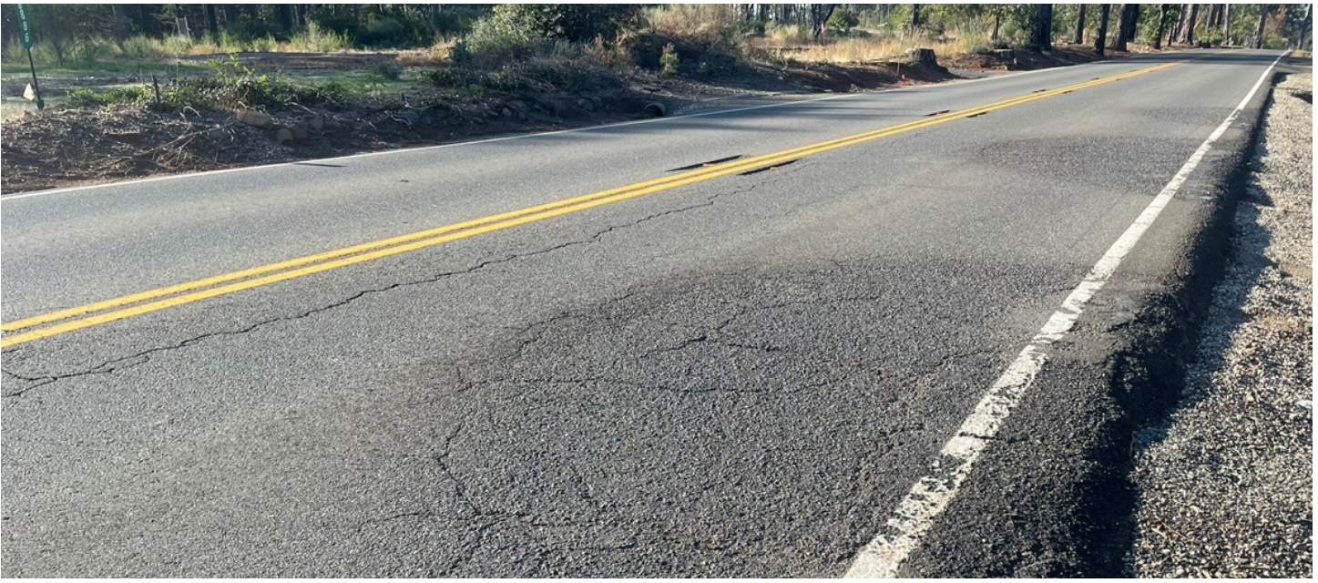
Figure 8. Photo. Cracking and raveling in burned area on Skyway Road in Paradise.
