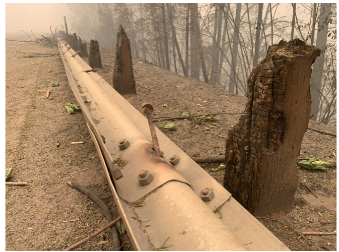
B. Guardrail post destruction.
