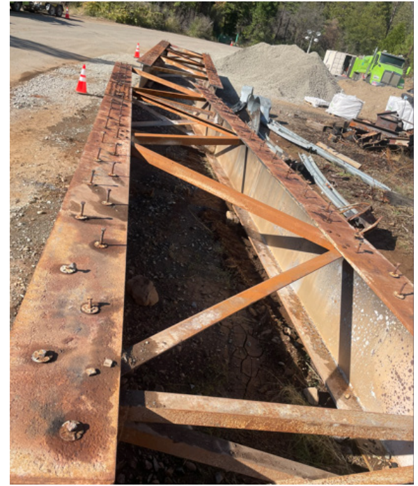
B. Recovered steel girder with intact cross bracing.
