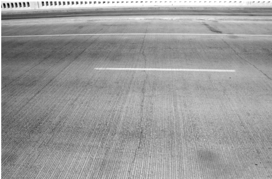
Figure 1.1: Transverse Cracking (Bridge 3)
