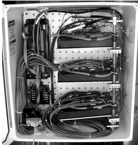
Figure 3.26: Datalogger System in Fiberglass Enclosure
