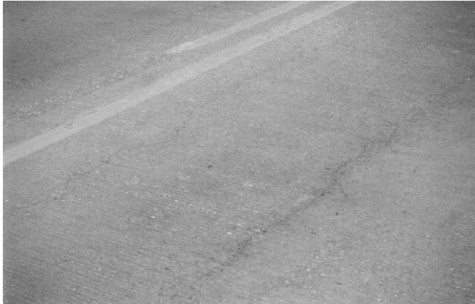
Figure A.20.3: Longitudinal Cracks in Bridge
