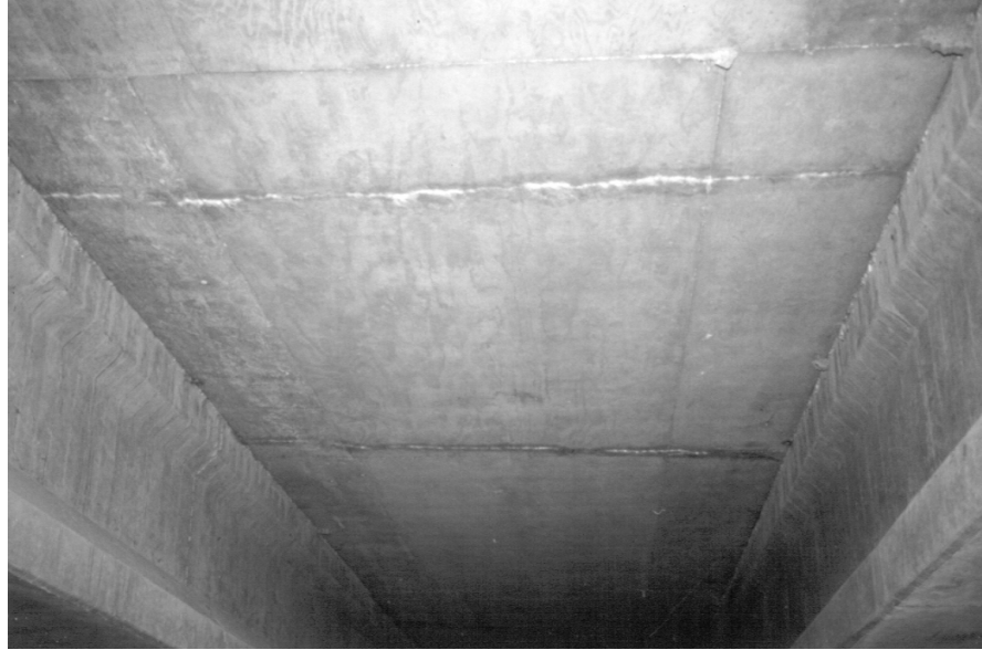
Figure 2.10: Transverse Cracks (Bridge 19)
