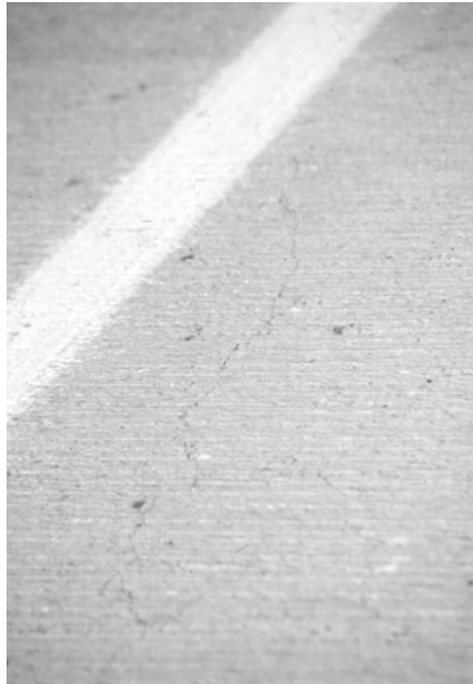
Figure 2.6: Longitudinal Crack near White Lane Edge Line (Bridge 1)
