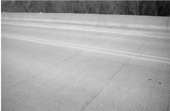
Figure A.7.3: Transverse Cracks on Bridge
