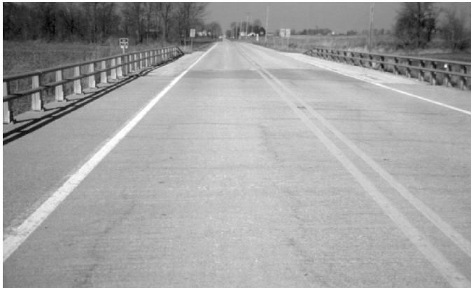
Figure A.8.2: Longitudinal Cracks on Bridge
