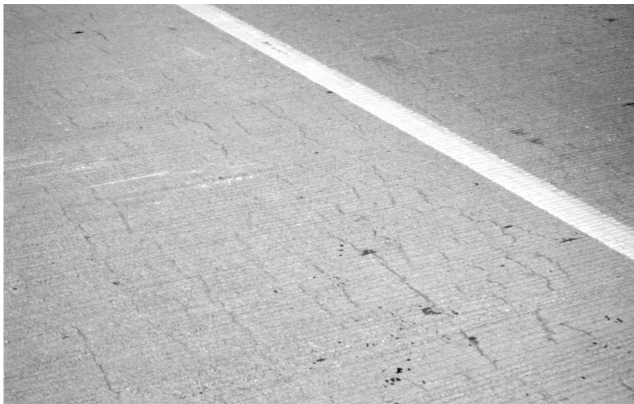
Figure 2.8: Map Cracking in Overlay (Bridge 6)
