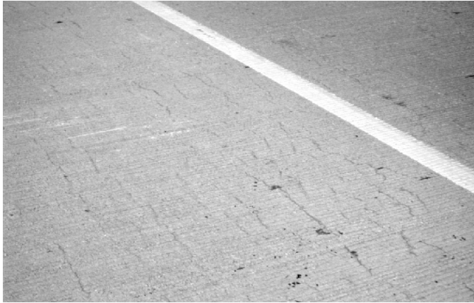
Figure A.6.1: Map Cracking in Overlay of Bridge
