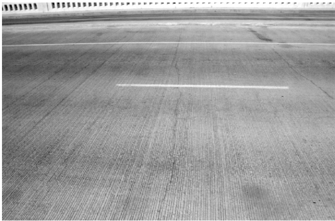
Figure A.3.3: Transverse Cracking in Bridge
