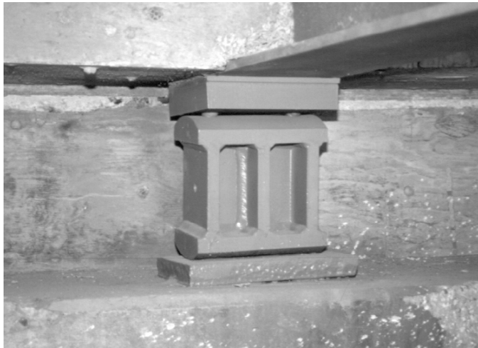
Figure A.4.2: Unseated Rocker Support for Steel I-Beam Girder of Bridge
