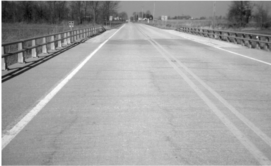
Figure 2.7: Longitudinal Cracks (Bridge 8)
