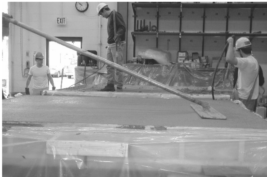
Figure 4.20: Bull Floating the Free-Shrinkage Model and Vibrating the Concrete in the As-Built Model
