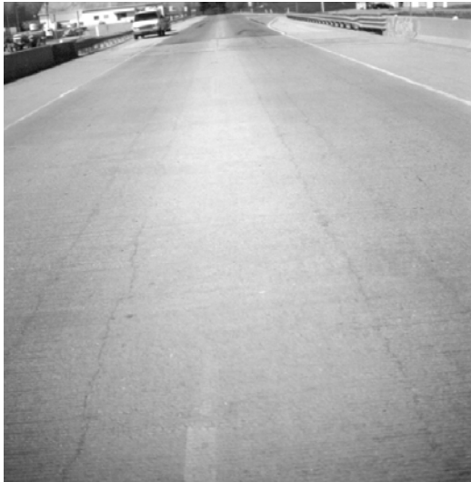
Figure A.18.2: Longitudinal Cracks in Bridge
