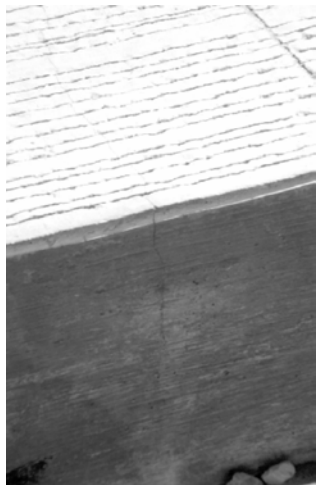
Figure A.14.4: Full Depth Longitudinal Crack at end of Bridge
