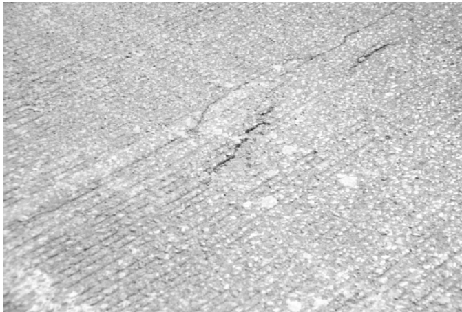
Figure A.9.2: Transverse Crack with Delamination on Bridge
