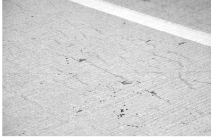
Figure 2.16: Map Cracking (Bridge 16)
