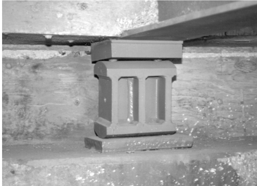
Figure 2.9: Unseated Rocker Support for Steel I-Beam Girder (Bridge 4)
