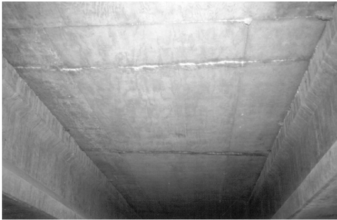
Figure A.19.2: Transverse Cracks in Bridge
