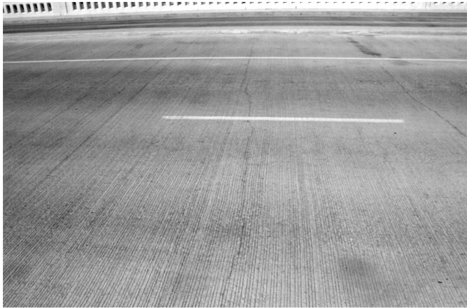
Figure 2.1: Transverse Cracking (Bridge 3)
