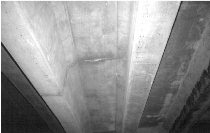
Figure A.12.2: Transverse Crack in Bridge
