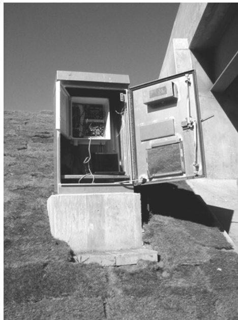
Figure 3.27: Datalogger System in M Cabinet
