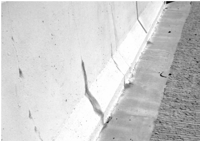
Figure A.2.2: Transverse Cracking in Bridge
