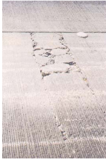
Figure 3-12: Punch-out on CRC Pavement [SHRP, 1993]
