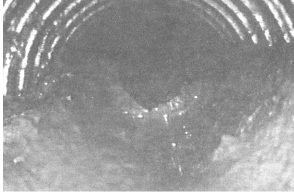
Figure 3-10: Silted Under-drain Pipes Identified by Video Inspection [Christopher And McGuffey, 1997]
