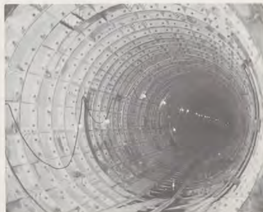
Massive steel rings form the inner surface of the tunnel running from the Nassif building (L'Enfant Station) to the Stadium-Armory Station in Northeast Washington. A single track runs in each tunnel.
