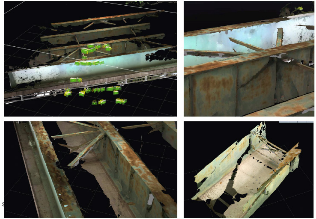
Figure 3.19 Summary of Field Implementation Testing Results at Davis Ferry Road Bridge. 3D Scanning Results.
