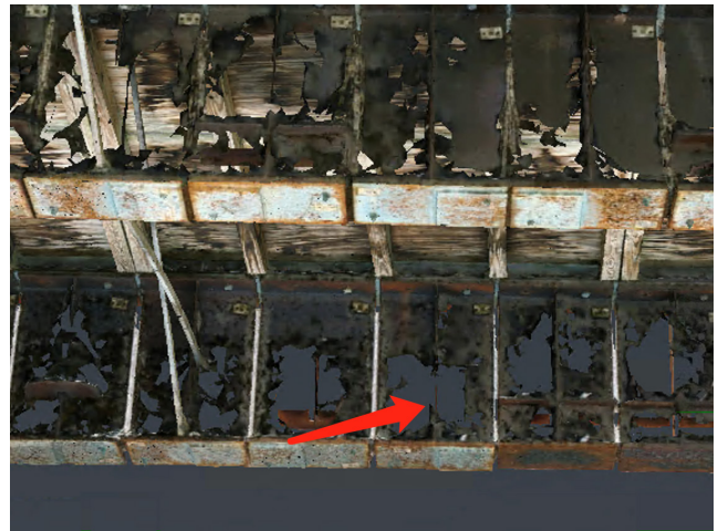
Figure 3.23 Incorrect Exposure and Resulting Incomplete 3D Model Sections: Lead Holes appearing in 3D Model.
