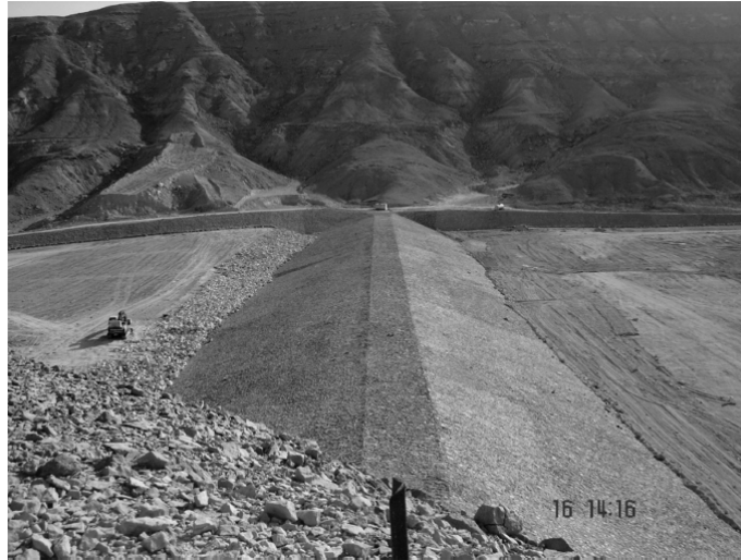
Figure B.30 Detention dam constructed across streams in an arid region (Wadi Watir, Egypt) to control flash floods (Soliman, 2010)
