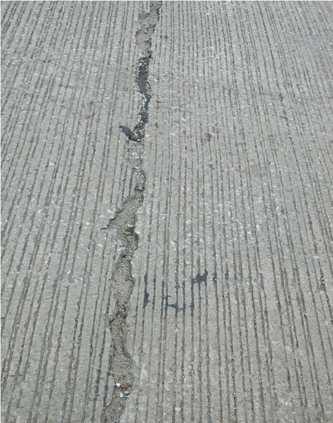
Unsealed Crack in Concrete Pavement – Notice exposed aggregate and opening in surface.
