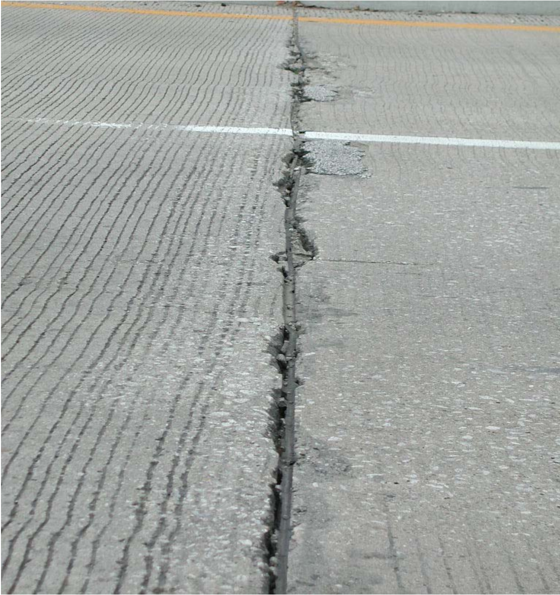
Bad Joint – The joint material has receded and there are gaps and spaces at the joint.
