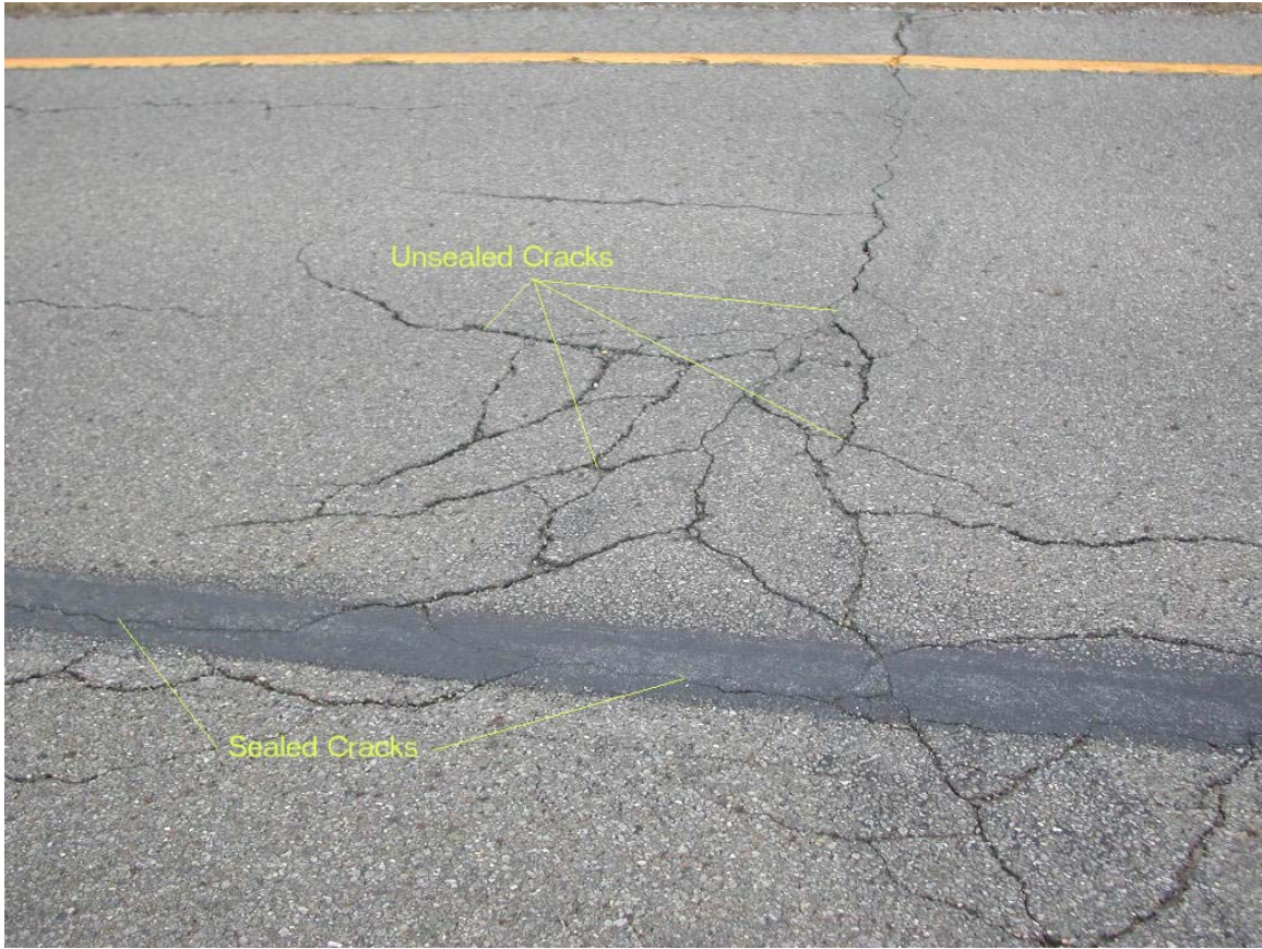
Asphalt Pavement – Sealed and unsealed cracks.
