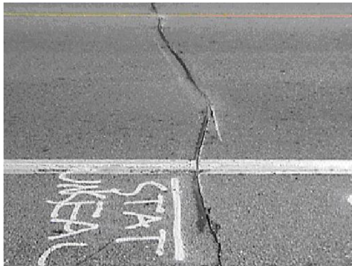
Figure 6-18 Routed Crack in Unsealed Section
