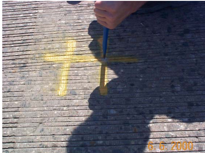
Figure 6-24 Marked Test Spot
