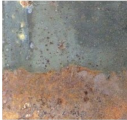
(b) 2012 rail (surface image of web)
