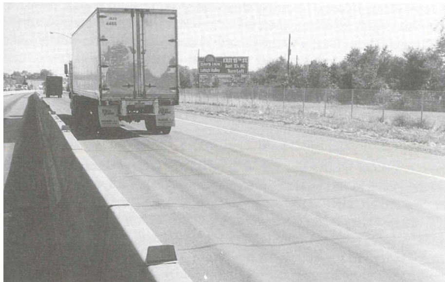
Figure 2.2 -- Rutting observed in an HMA pavement (4)
