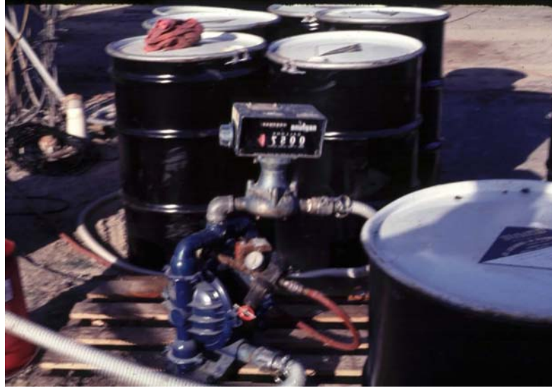
Figure 12 Meter Used to Control Flow of SBR into Plant
