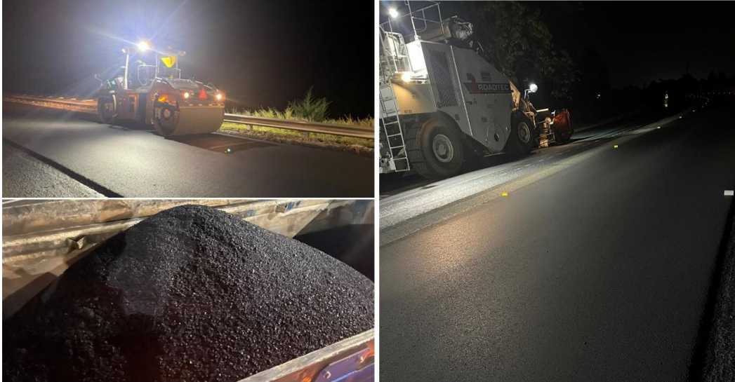
Figure 5. Production, Paving Operations, and Placement of Mixture with High Content of Reclaimed Asphalt Pavement and Recycling Agent RA2
