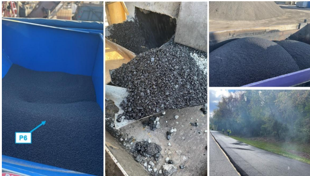
Figure 3. Production, Paving Operations, and Placement of Recycled Plastic-Modified Mixture with Plastic Additive P6
