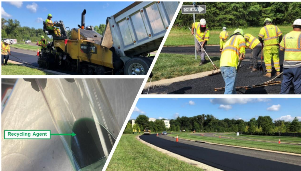
Figure 4. Production, Paving Operations, and Placement of Mixture with High Content of Reclaimed Asphalt Pavement and Recycling Agent RA1
