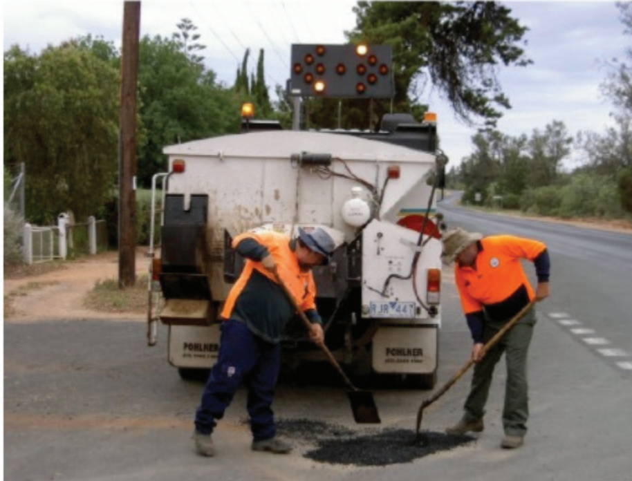
Figure 1.1 Road Patching With a Patching Truck [From Local Government & Municipal Knowledge Base by Mildura Rural City Council CC BY-SA 3.0].
