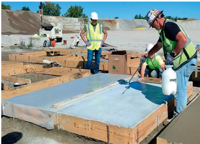
Figure 6.10 Application of a Spray-On Curing Compound to Half of Slab #6 (REF) and #8 (REF+Slag). The Plastic Sheet on the Other Half of the Slab Was Removed After Spraying.
