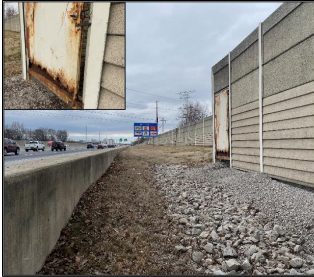
Figure D.6 Fire access door in noise barrier along I-465, West of Indianapolis, IN. Inset: Close-up of rusted door bolted shut.
