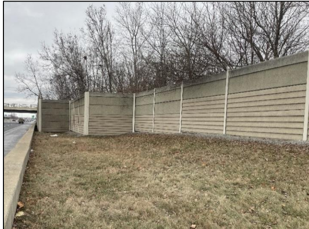
Figure D.7 Elevated roadside behind barrier wall with woody vegetation growing over noise barrier along I-465 Indianapolis, IN.
