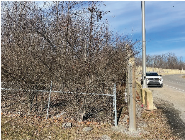
Figure 2.4 Noise Barrier With Vegetation Growth Over Wall and Access Difficulty Along I-465.
