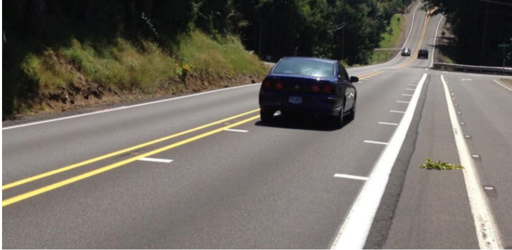
Figure 3.23 Optical Speed Bars (UDOT, 2023b)
