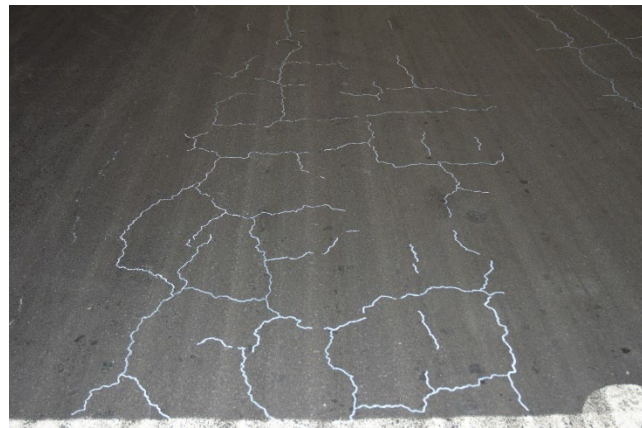
(b) Area of alligator cracking
