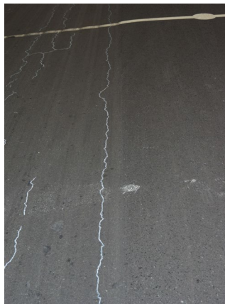
(a) Linear crack at edge of traffic area
