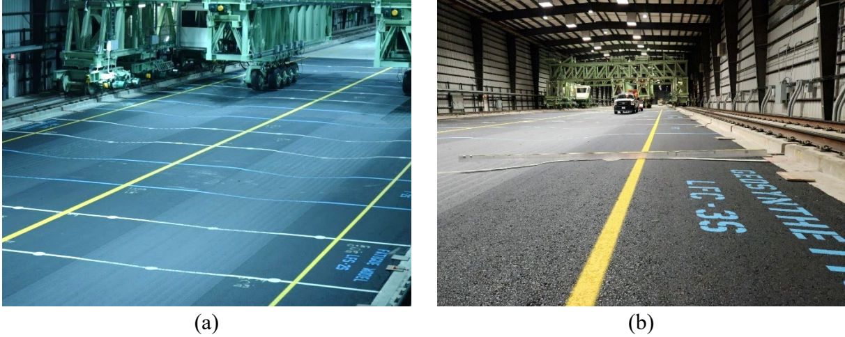
Figure 37. Final Surface Condition of Geosynthetic Test Items: (a) View Facing Northeast Toward the Geosynthetics Test Area Showing Heavily Deformed Surface (November 8, 2022) and (b) Upheaval, Test Item LFC-3S (November 3, 2022) (The trafficked area is on the left. The shoulder was initially level with the curb [right].)
