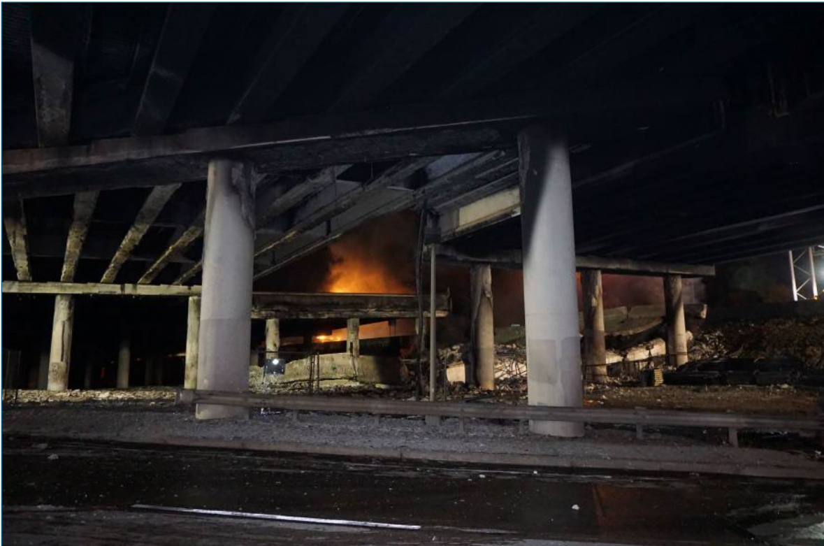
Figure 9. Photo. Atlanta Interstate bridge failure [119].
