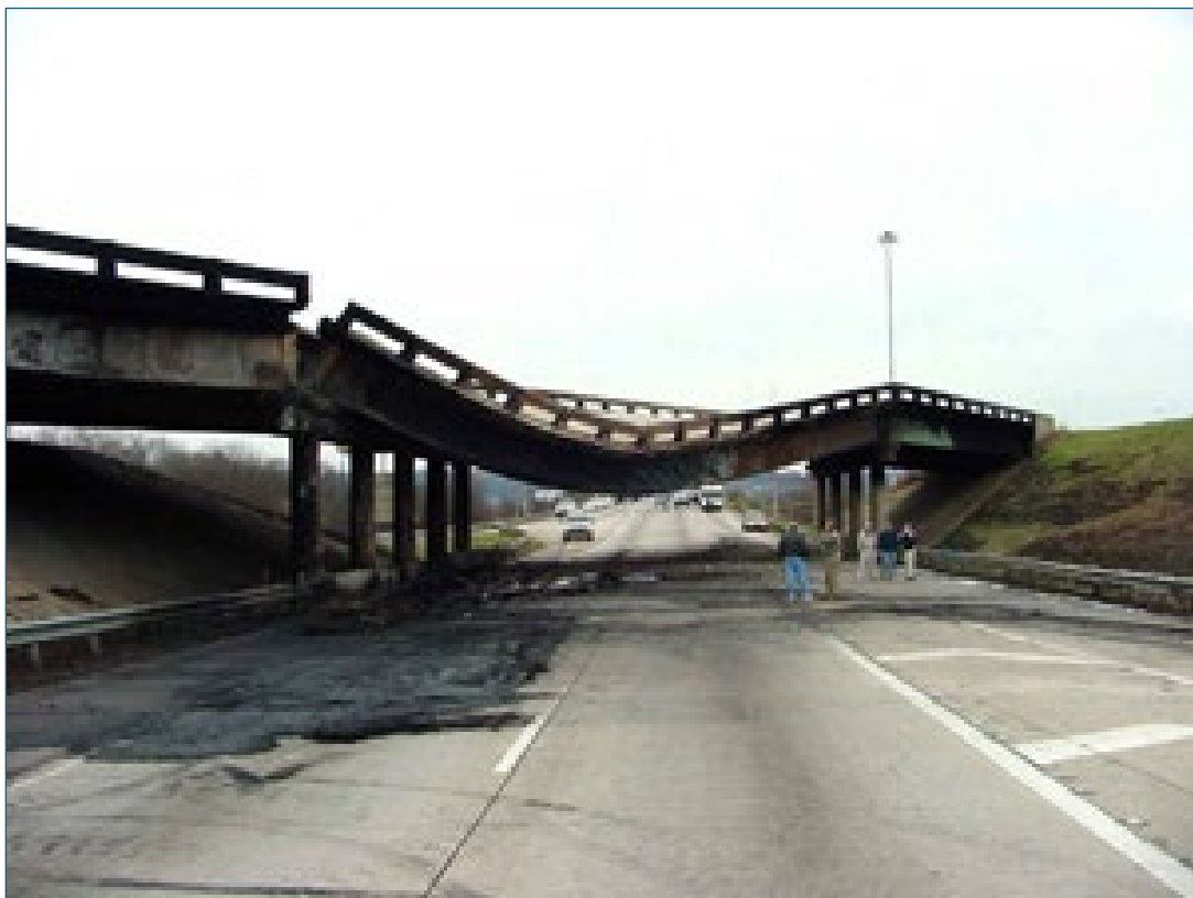
Figure 6. Photo. Malfunction Junction 2002 post-fire [94].
