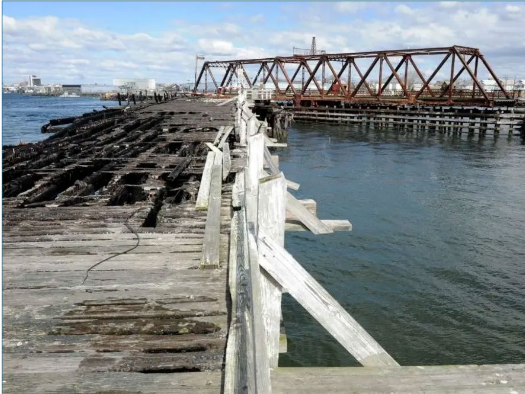
Figure 4. Photo. Pleasure Beach Bridge post-fire [78].
