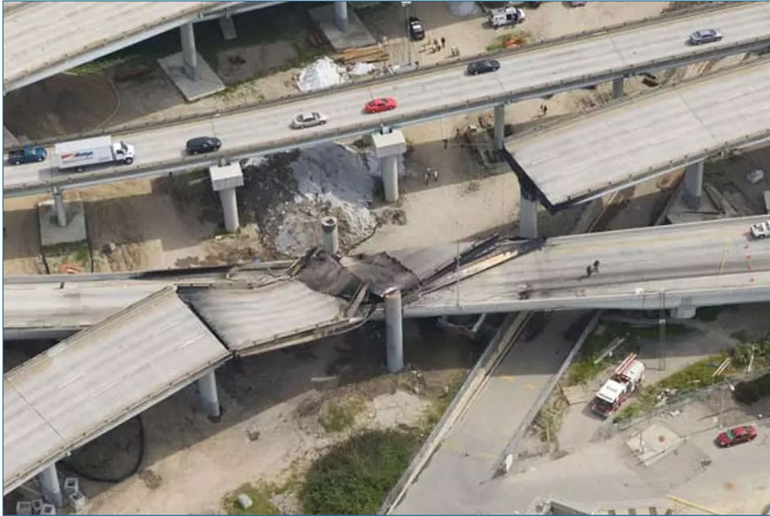
Figure 7. Photo. MacArthur Maze post-fire [108].
