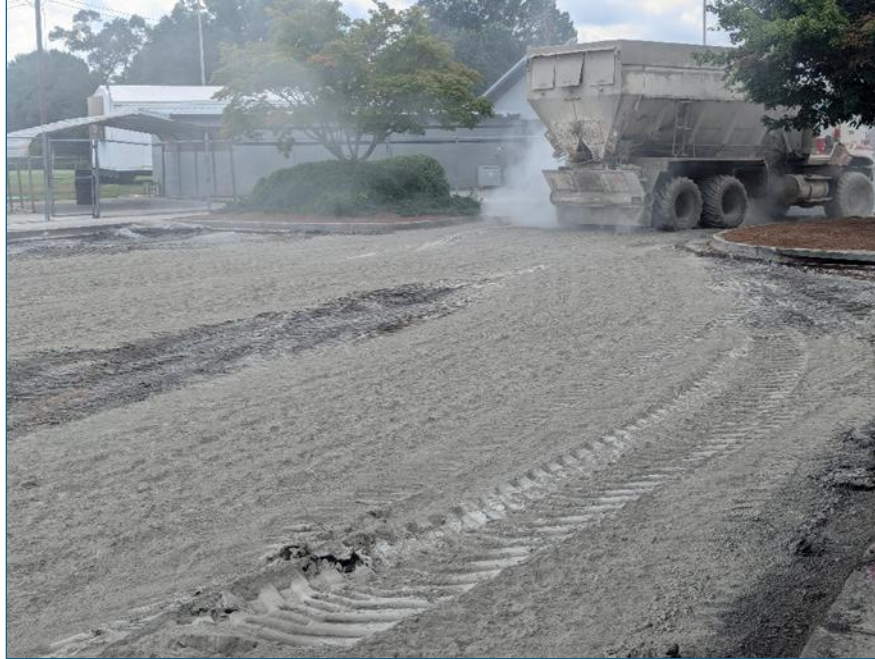
Figure 2. Photo. Cement application by a spreader truck on an FDR construction site.
