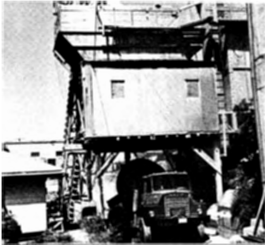
Photograph 1: Concrete batch plant used to produce the base lift and the wax bead concrete.
