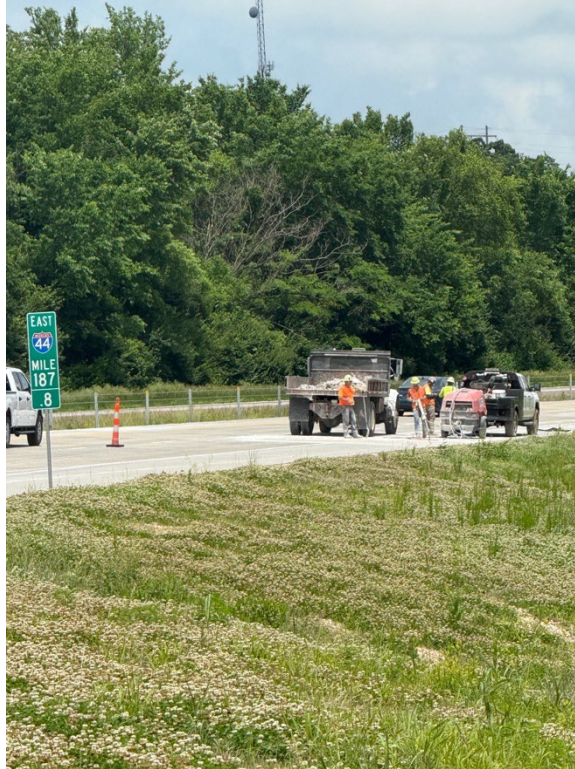
Figure 7-1. Workers and equipment in closed lane on I-44 near Rolla and St. James.
