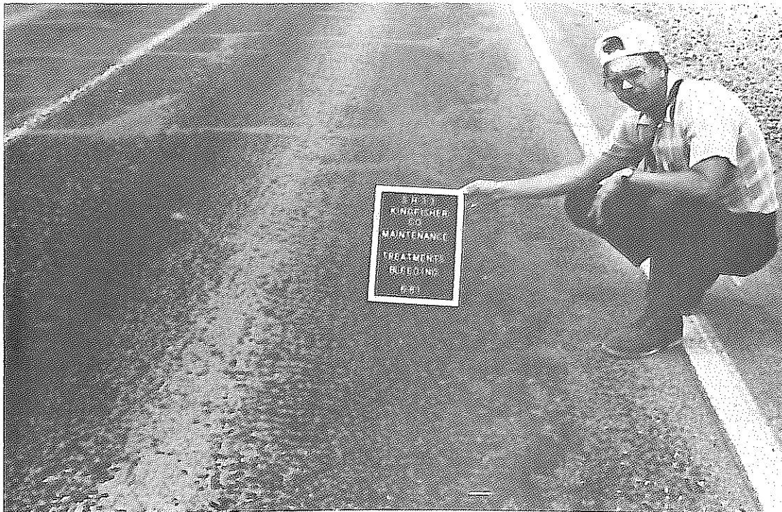
Figure 1B. The flushed condition of the surface prior to Asphalt-Rubber treatment.
