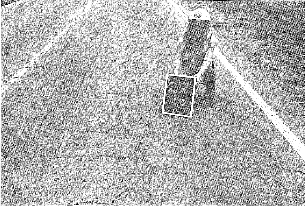
Figure 1A. The cracked condition of the surface prior to the Asphalt-Rubber treatment.
