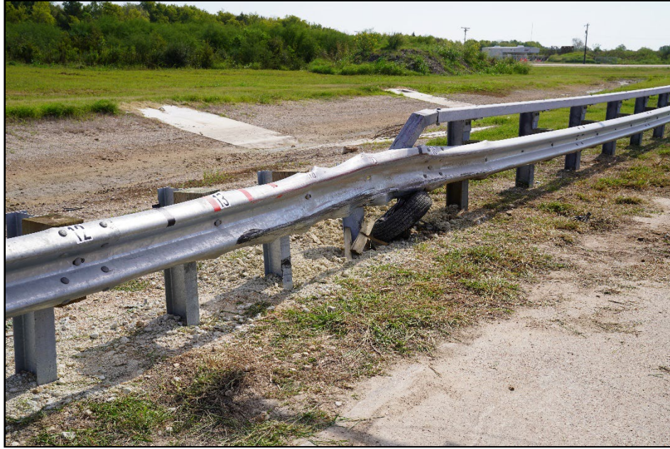
Figure 6.5. Transition after Test at Impact Location for Test 441203-01-1.
