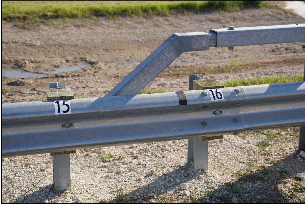
Figure 3.4. TL-4 Test Installation at the Transition Box Beam Rail prior to Testing.
