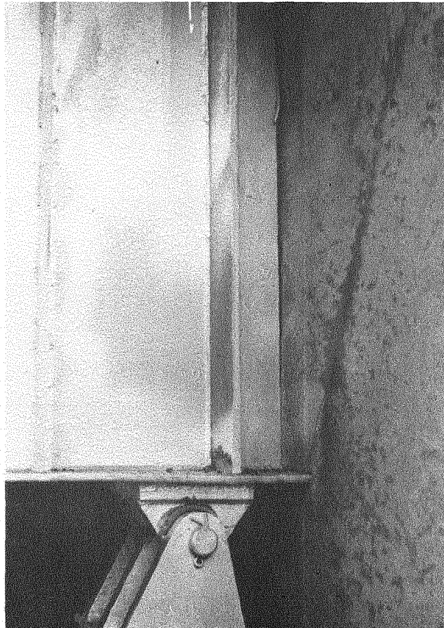
Fig. 2-15. Evidence of extensive movement of abutment headwall
