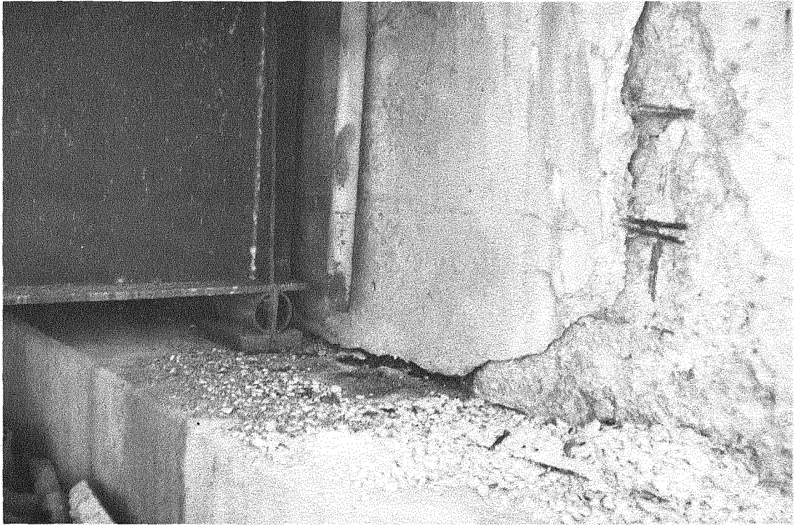
Fig. 2-19. Expansion device showing minor tilting
