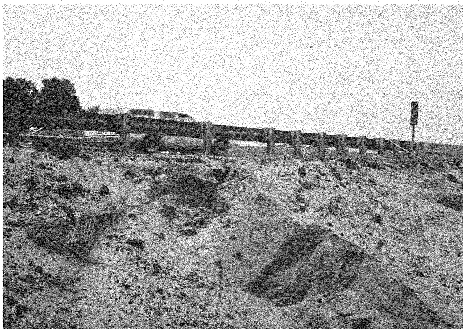
Fig. 2-11. An approach embankment showing erosion
