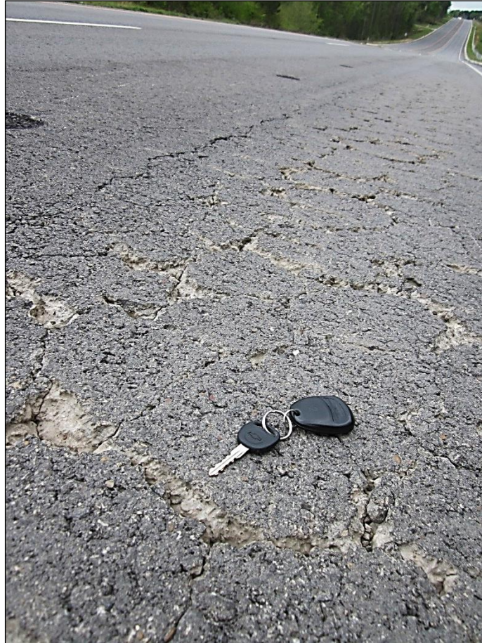
Figure 60. Premature Fatigue Cracking, Project 3.
