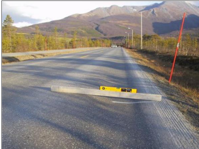
Figure 10. Settlement of a Widened Road Shoulder over Peat Soil in Norway (6).
