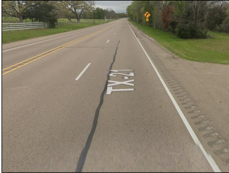
Figure 2. Longitudinal Crack in a Widened Pavement.
