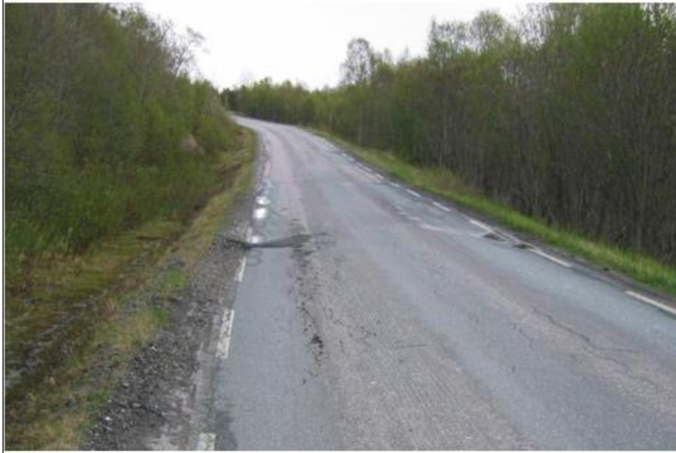
Figure 11. Edge and Drainage Failure (6).
