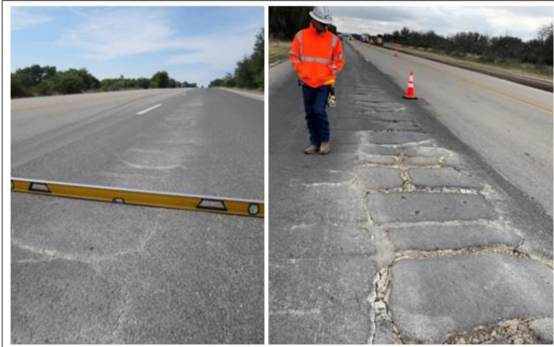
Figure 8. Failure of US 83 on Inside Lane.
