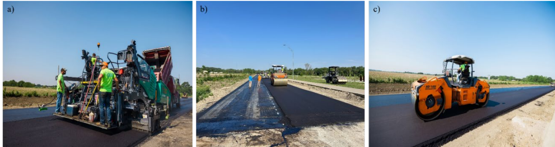
Figure 3.11 Field implementation: (a) Paving; (b) compaction of SPR_RAP25 (plant-produced); (c) compaction of SPR_RAP25_LDPE 2 (plant-produced).
