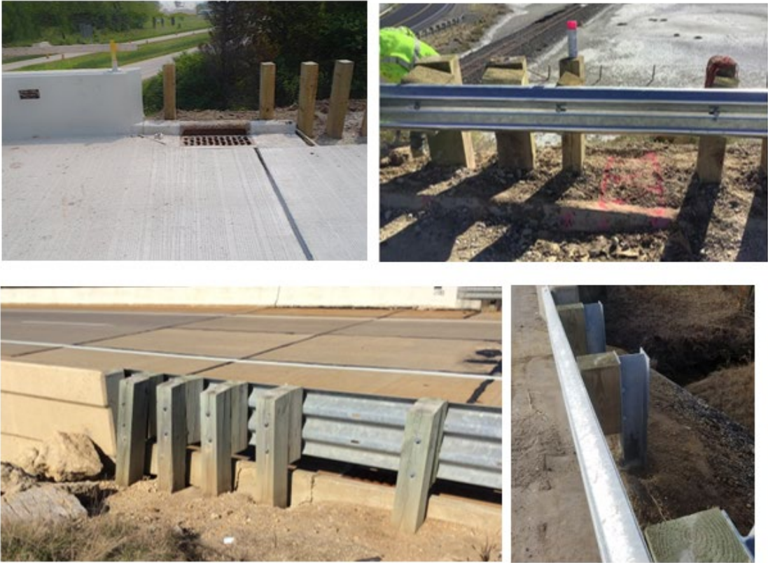
Figure 1. Typical example of obstructions and site constraints near concrete bridge rail ends
