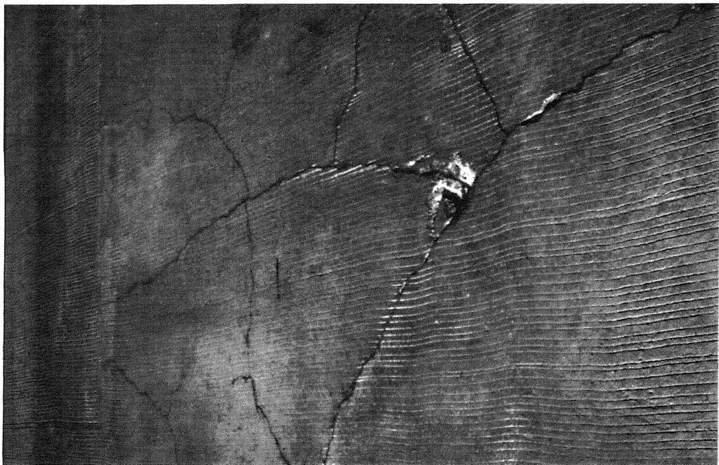
Figure 10. Severely Cracked Section(close-up).
