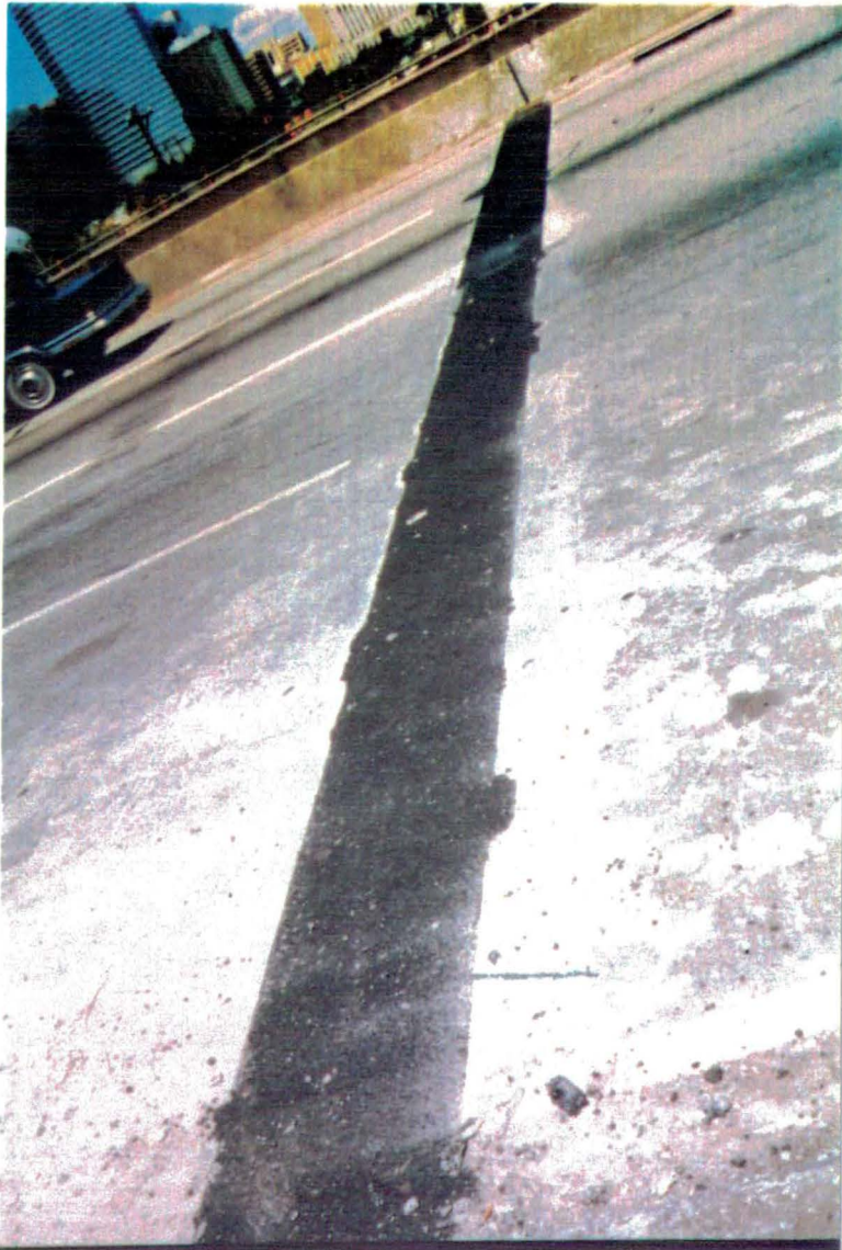
Figure 14. Completed KOCH BJS Unit.
