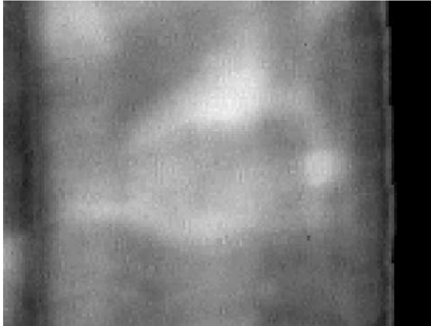
Figure 7 - B670122 - Aerial Delamination - Defect #2 - 1,000 Feet Above Deck
