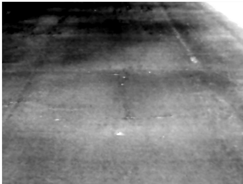
Figure 4 - B670122 - Handheld Delamination - Defect #2
