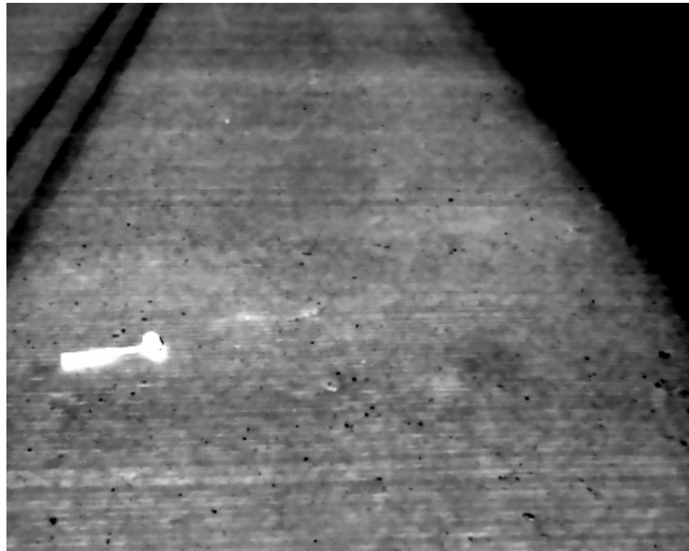
Handheld IR Camera (hammer indicating one of the defects)
