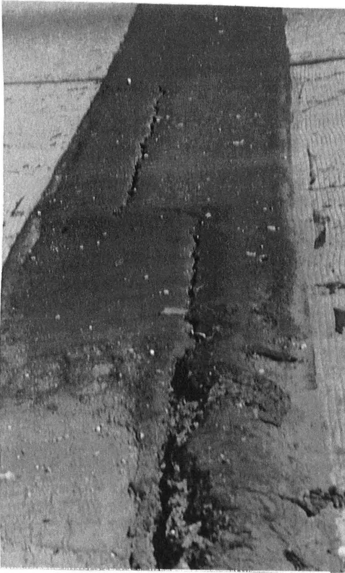
Figure 7. Cracked BJS Unit, 7-10-92.
