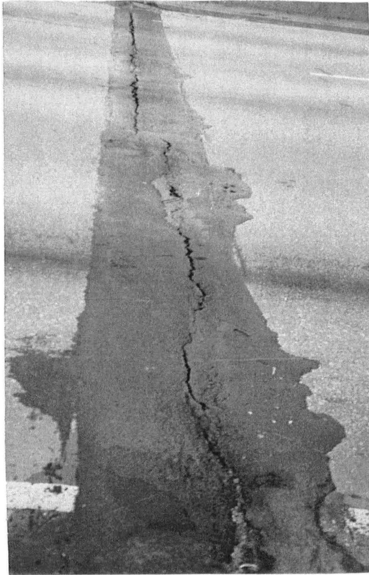
Figure 9. Typical cracked BJS Unit, March 4, 1993
