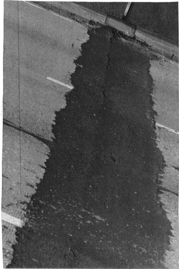
Figure 8. Cracked BJS Unit, 7-10-92.
