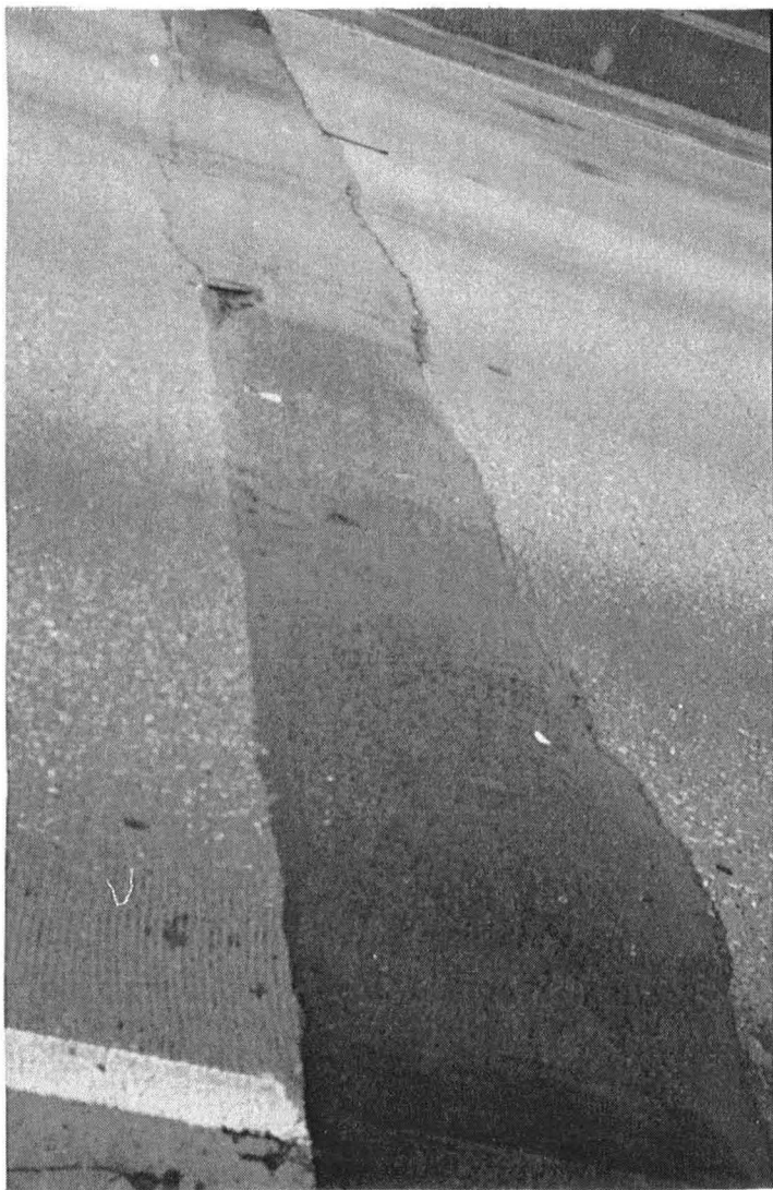
Figure 11. Spalling at edge of BJS Unit, March 4, 1993
