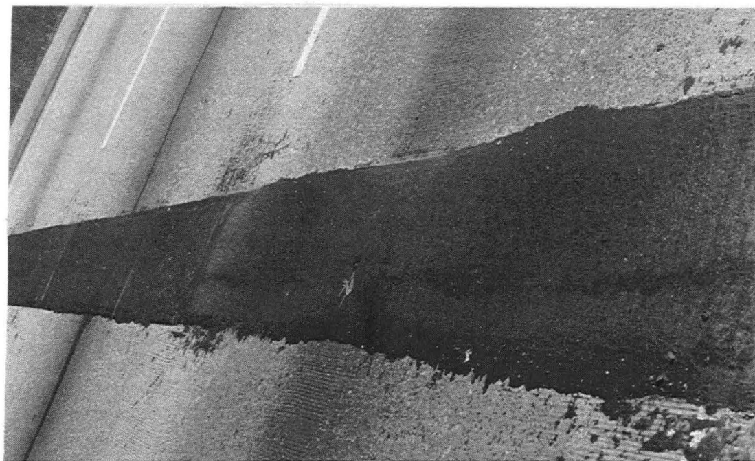
Figure 5. BJS Unit with "healed" crack (depressed area).
