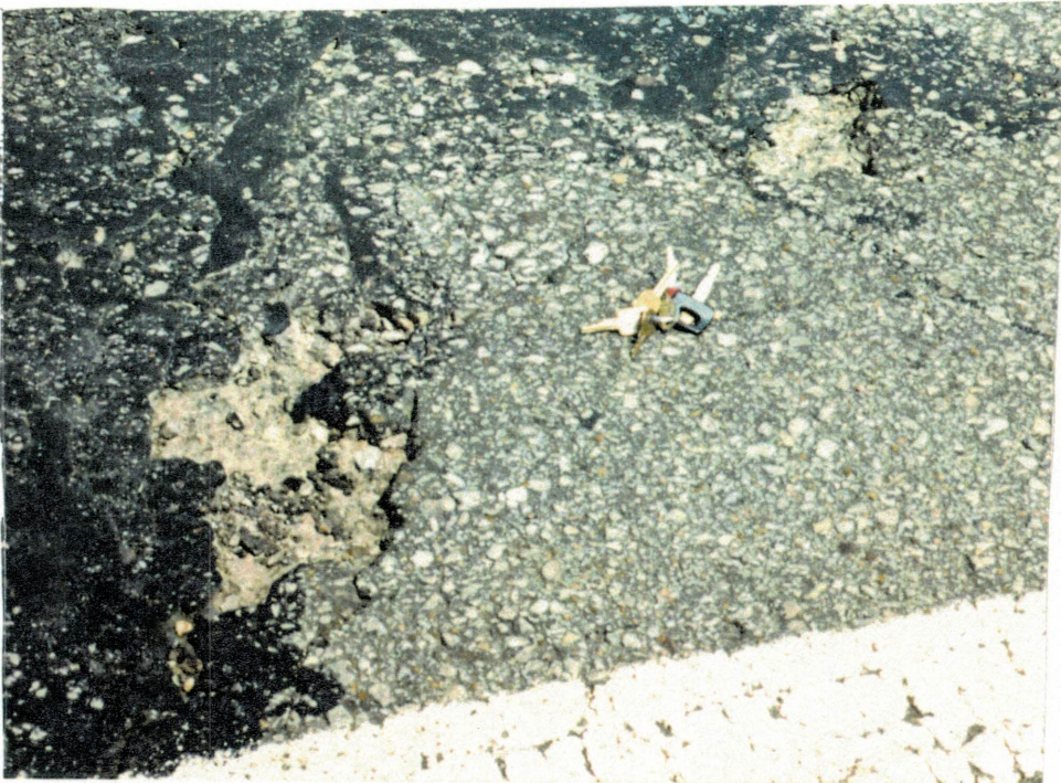
Figure 6. Area at Intersection of Cracks with Surface Pavement Layer Spalled Away.
