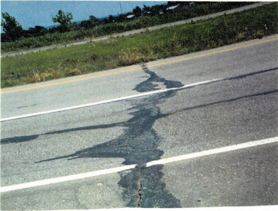
Figure 5. Typical Depressed Transverse Crack.
