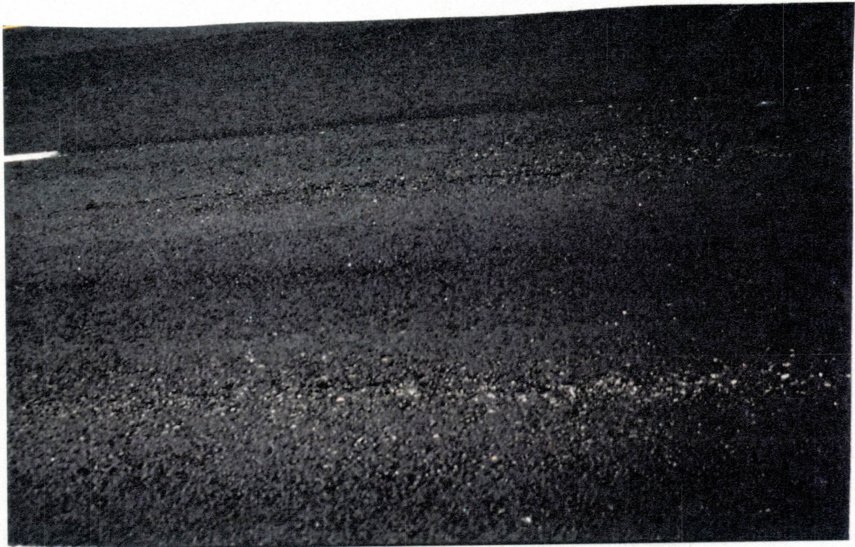
Figure 20. Typical Cracking in AC-40 Section.
