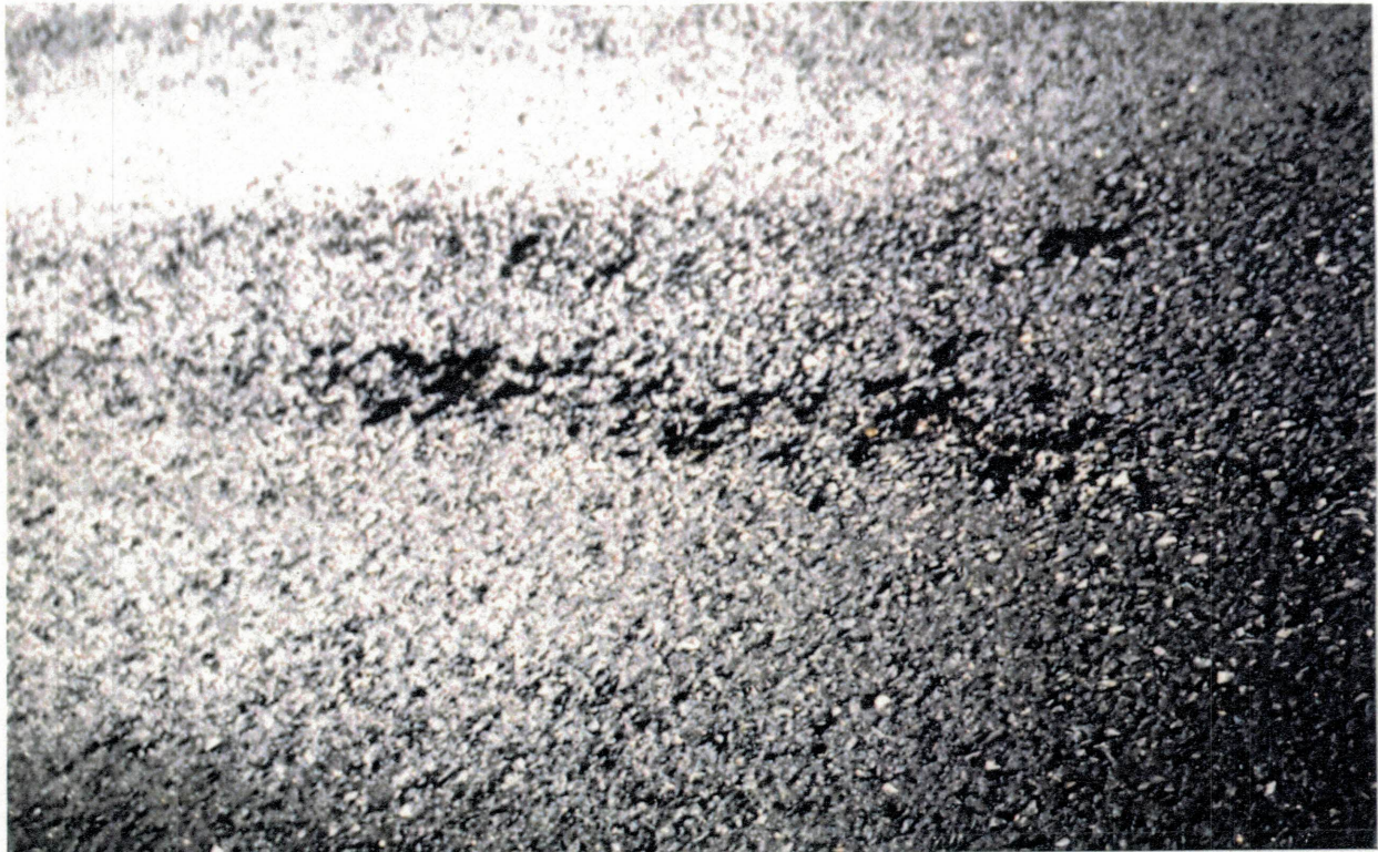
Figure 21. Ravelling of Aggregate From Surface Course.
