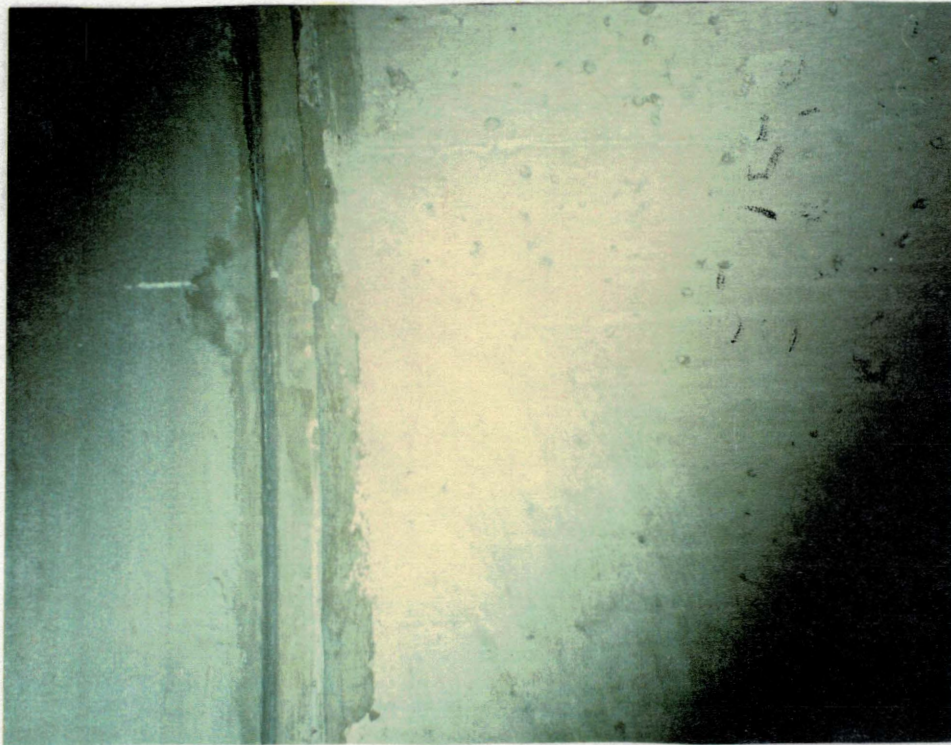
Figure 8. RCP Joint Patched With Mortar.
