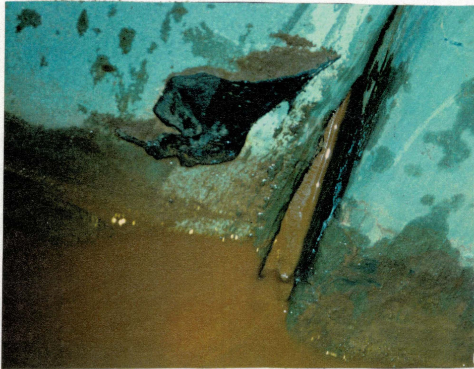
Figure 6. Leaking Joint in 2.4 m (96 in) RCP.
