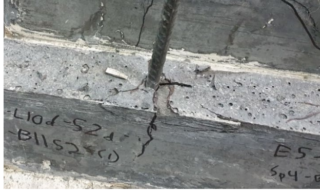
Figure 3.2: Splitting Cracks on Pullout Specimen
