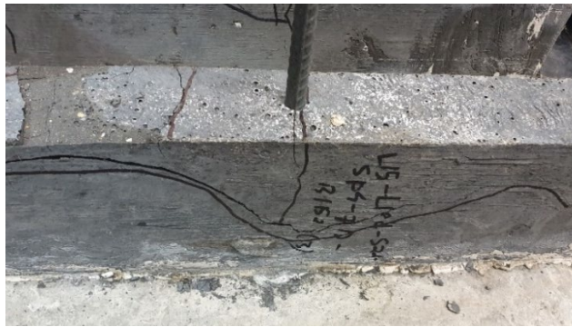
Figure 3.3: Open Diagonal Cracks on Pullout Specimen
