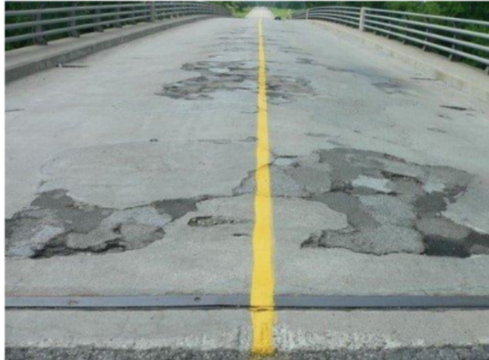
Figure 1 Significant Deterioration in a Concrete Bridge Deck [3]
