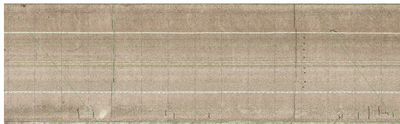
Figure 79 Existing Cracks on Bridge Deck No. 22451-Span 2
