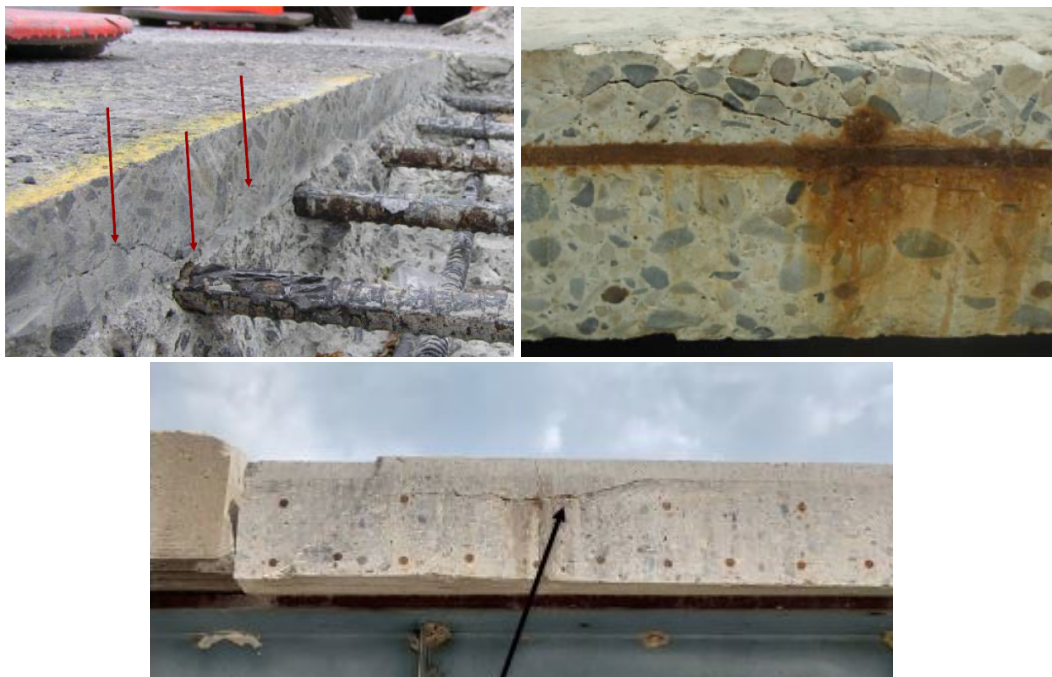
Figure 3 A slab with Naturally Occurring Delamination [6], [7], [8]
