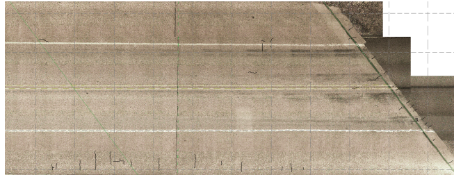
Figure 80 Existing Cracks on Bridge Deck No. 22451-Span 3
