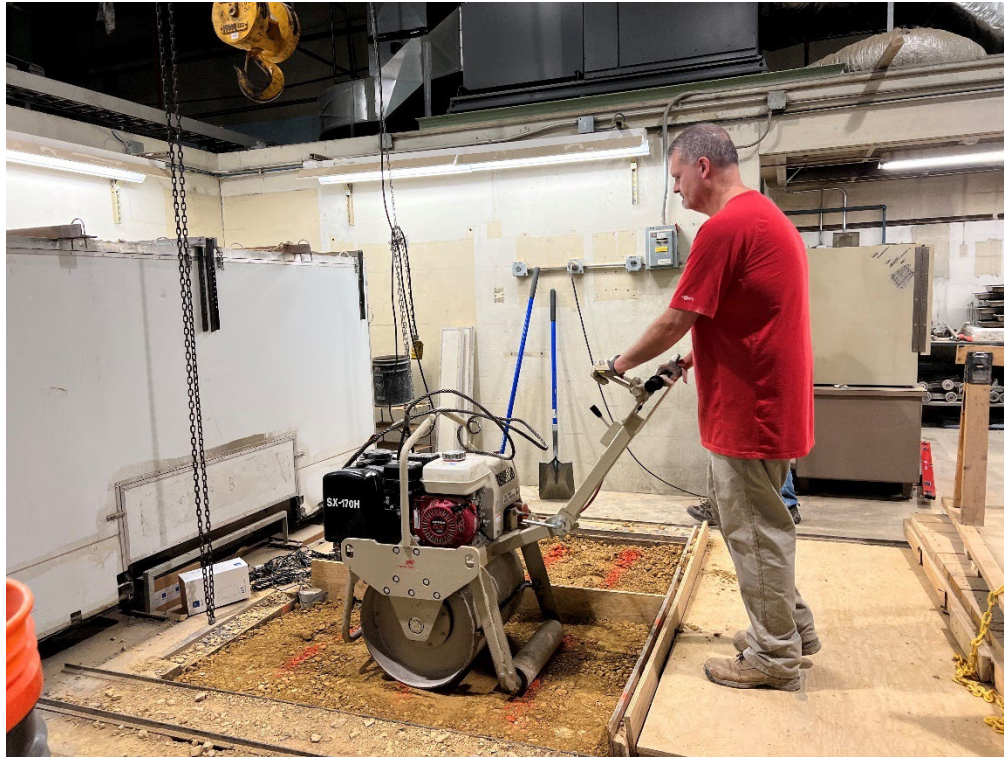
Figure 43. Using a vibratory roller for compaction of the soil inside the pit
