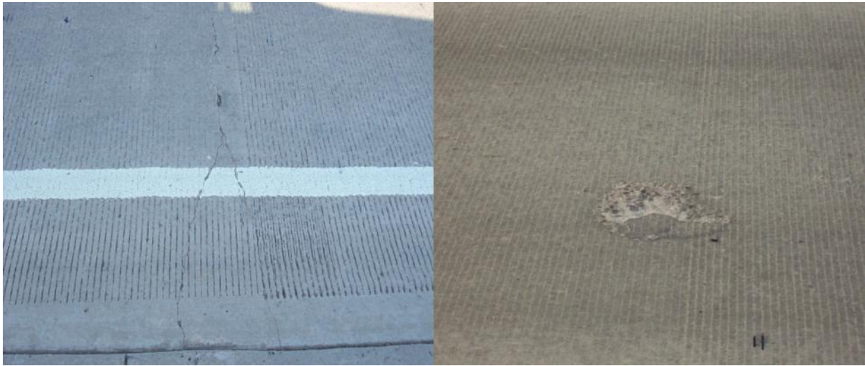
Figure 3.15 – (Left) Typical Y-crack for the region, (right) circular spalled area
