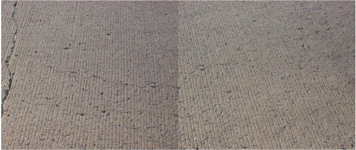
Figure 3.67 – Map cracking in the south bound lane
