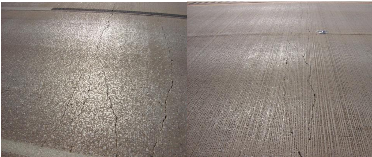
Figure 3.3 – Photo shows Y-cracks with multiple branches
