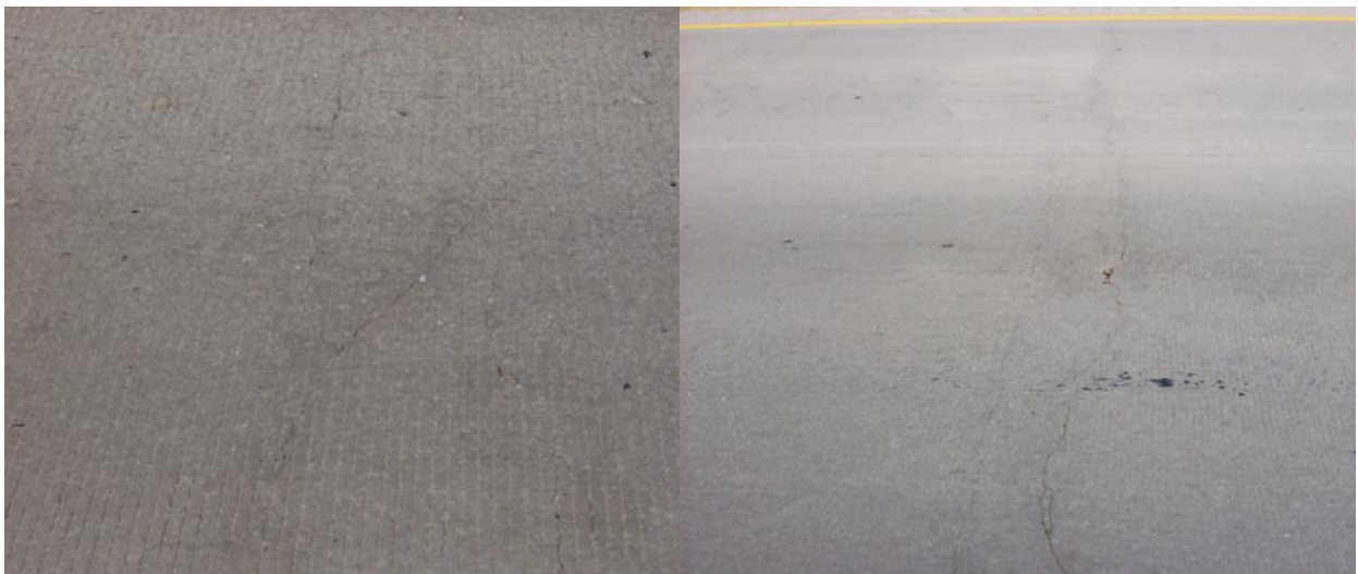
Figure 3.17 – (Left) Y-crack located in the region; (right) two close transverse cracks showing distress
