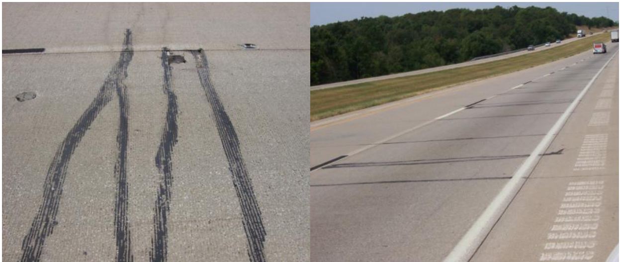
Figure 3.29 – Transverse cracks sealed with an asphalt joint sealant
