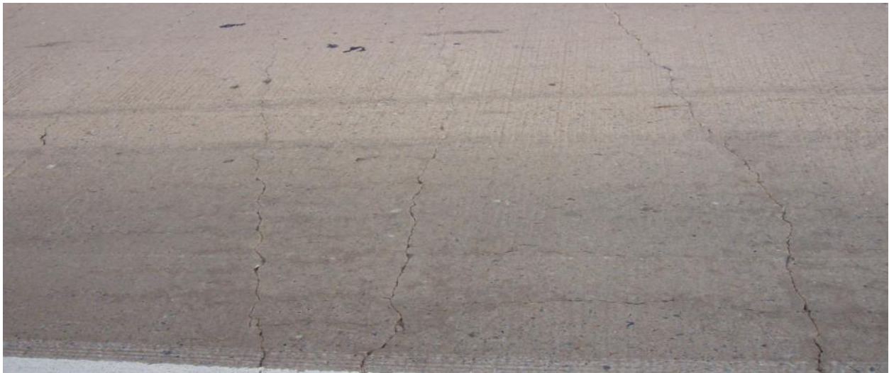
Figure 3.55 – Stretch of pavement showing signs of map-cracking
