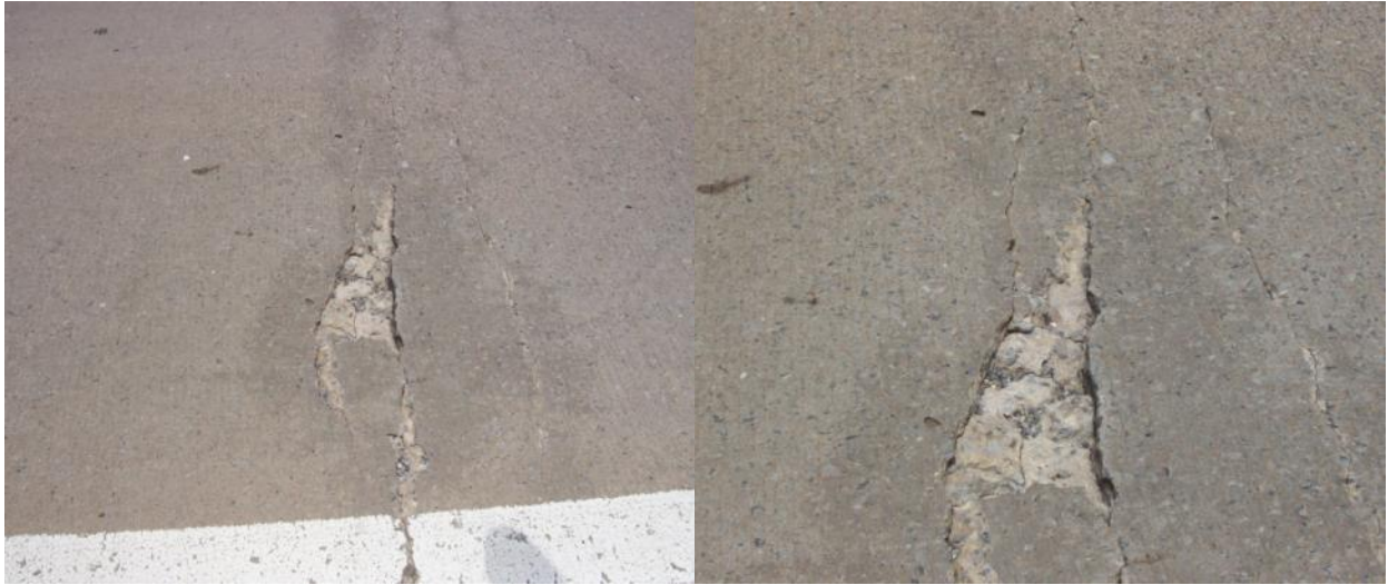
Figure 3.62 – Y-crack developing into a punch-out
