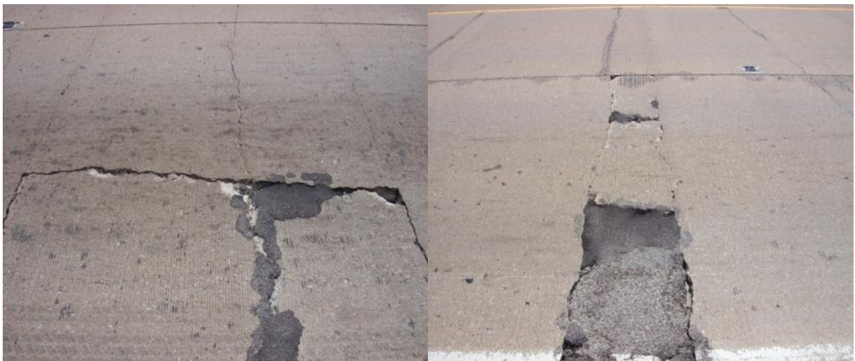
Figure 3.47 – Transverse cracks intersected by longitudinal cracks
