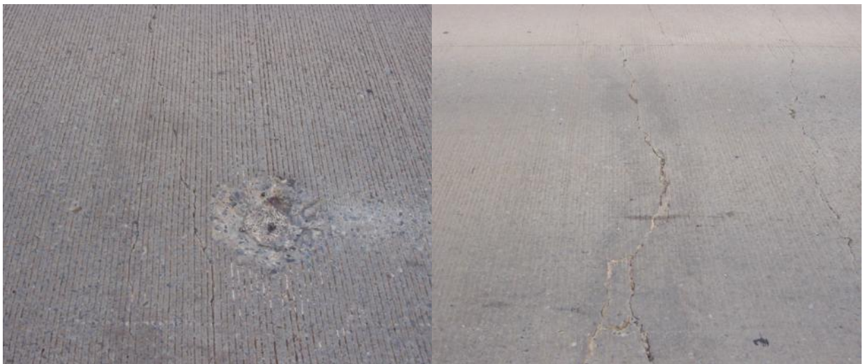
Figure 3.53 – (Left) Large circular distress, (right) Spalled Y-crack beginning to break up
