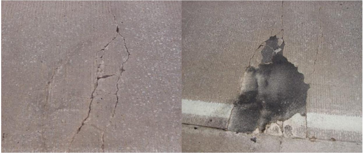
Figure 3.24 – Two instances where a Y-crack seemed to be developing into a punch-out
