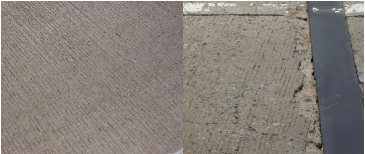
Figure 3.65 – Close ups showing map-cracking
