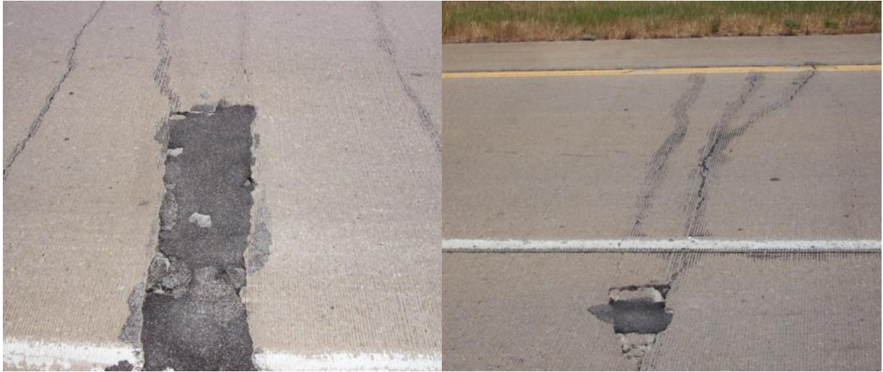
Figure 3.50 – Patches that appear to be the result of a failed Y-crack
