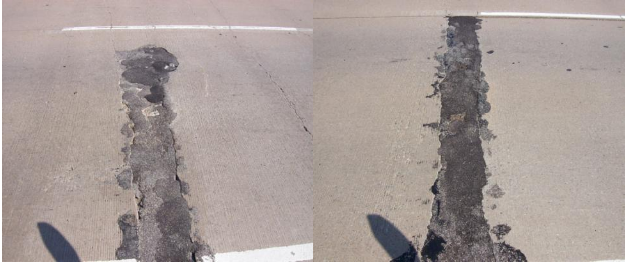
Figure 3.41 – Patches caused by closely spaced transverse cracks
