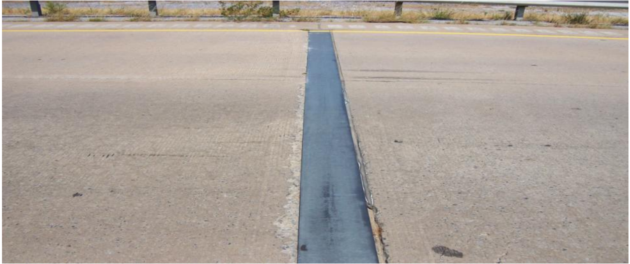
Figure 3.39 – Spalled terminal joint with worn roadway surface
