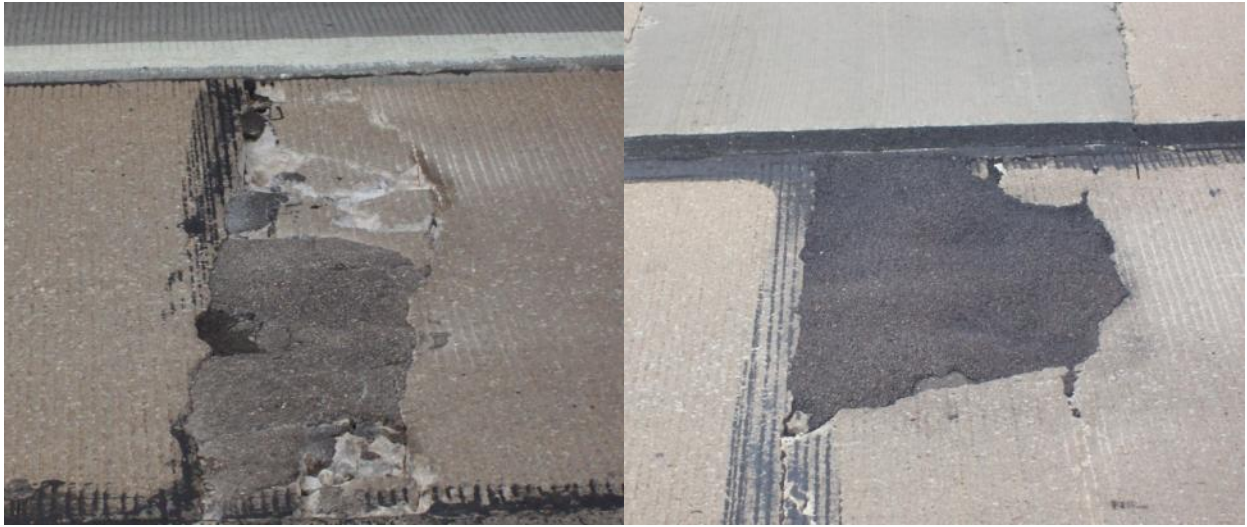
Figure 3.28 – Patches caused by closely spaced transverse cracks
