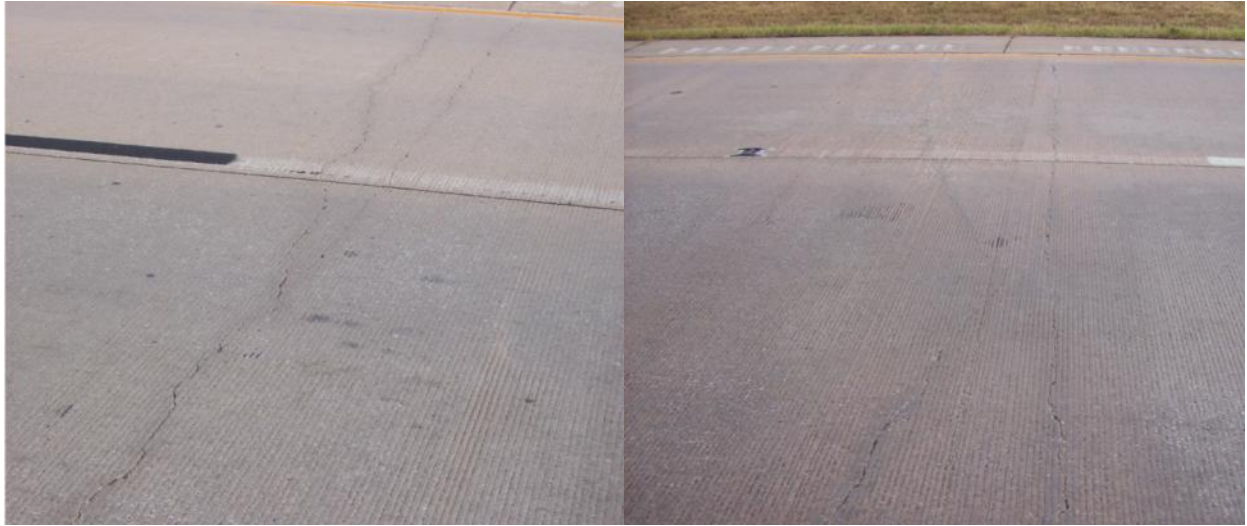
Figure 3.22 – Two different types of Y-cracks found in the area
