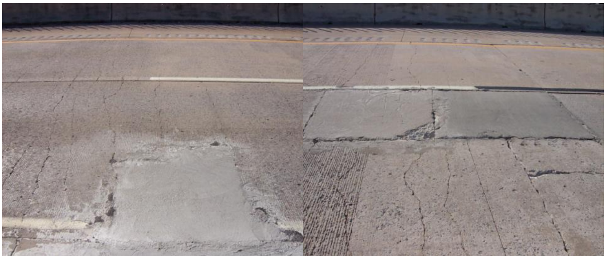
Figure 3.64 – Patches formed near closely spaced transverse cracks
