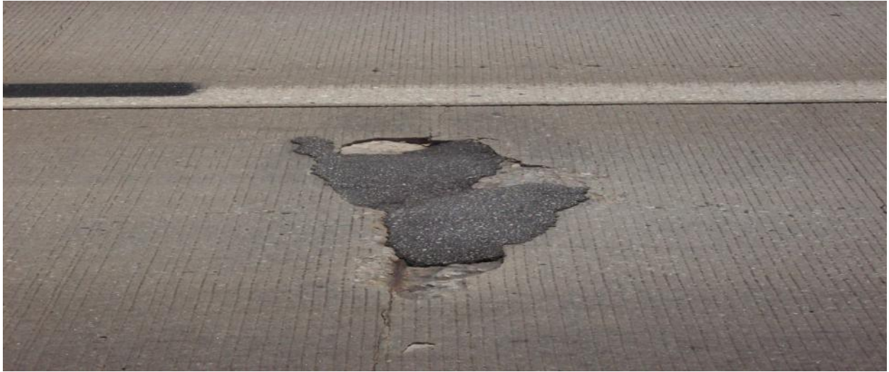
Figure 3.10 – AC patch over a distress with exposed transverse steel
