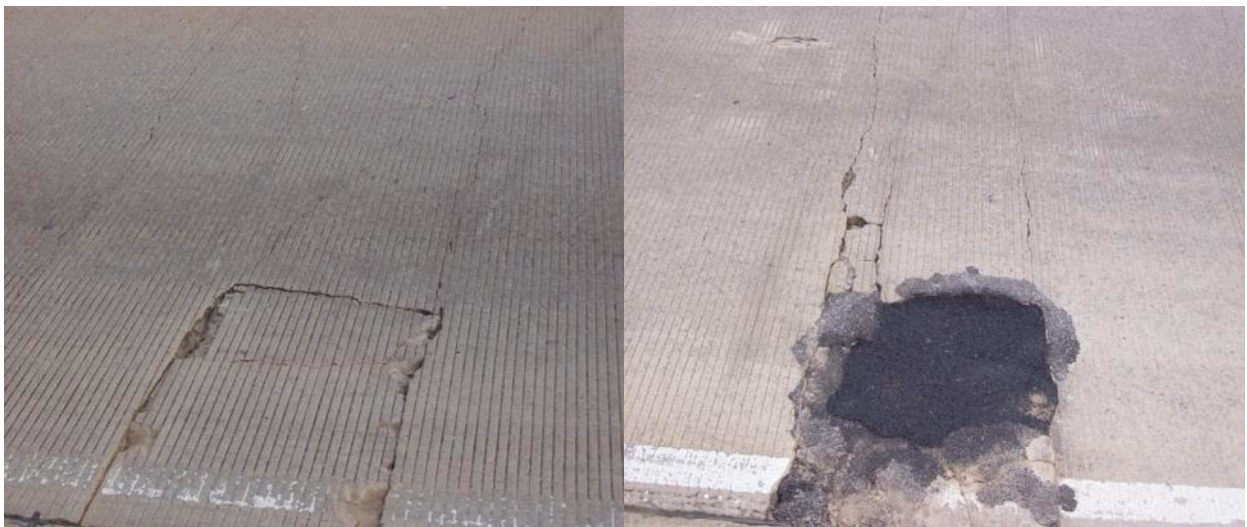
Figure 3.36 – Y-cracks leading to punch-out and eventually failure
