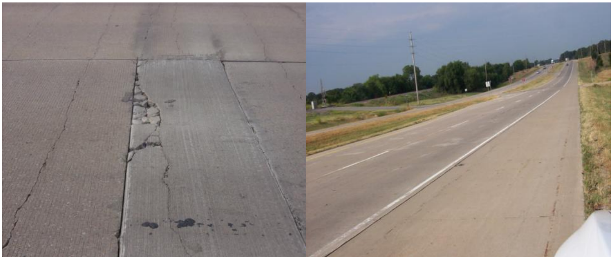
Figure 3.38 – (left) patch showing signs of distress (right) area of road where crack survey was taken
