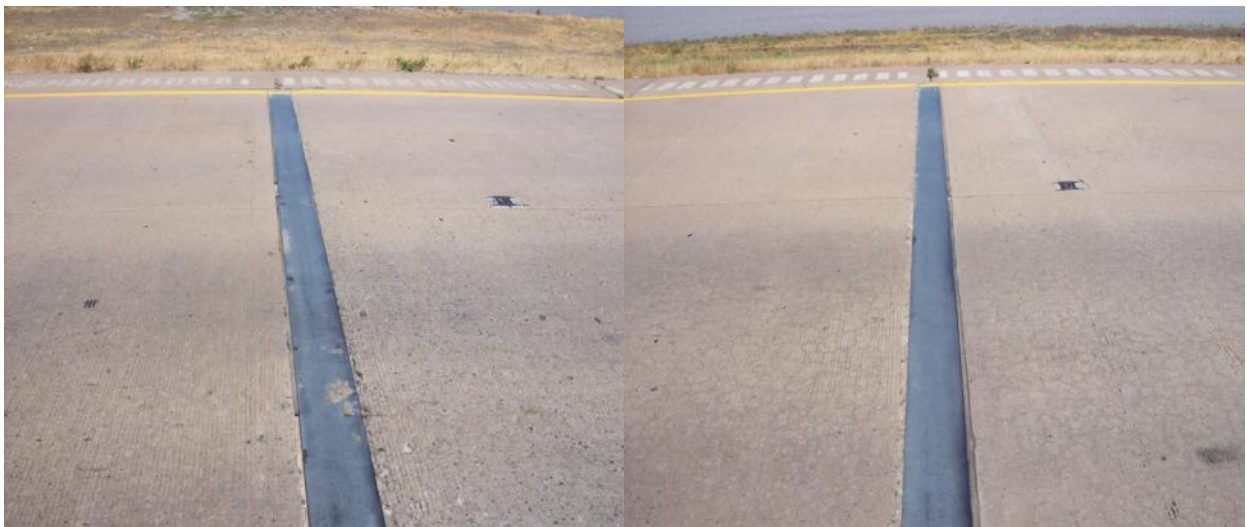
Figure 3.40 – Spalled terminal joints, with the (right) displaying map-cracking
