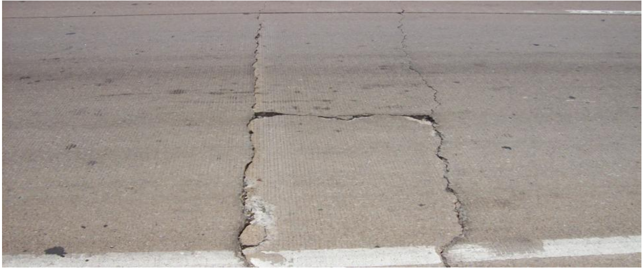
Figure 3.48 – Two transverse cracks intersected by a longitudinal crack
