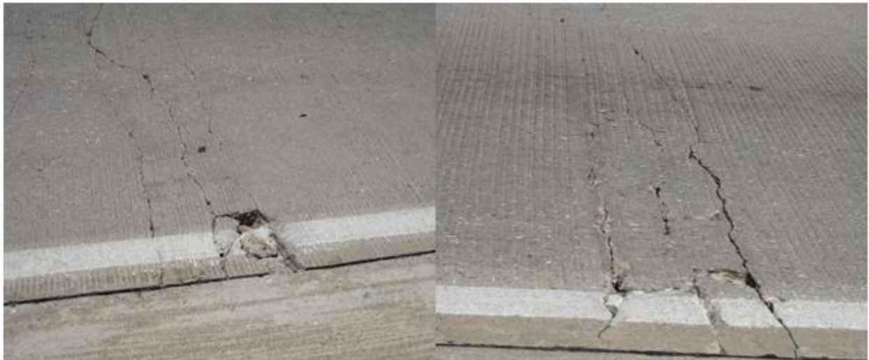
Figure 3.5 – Developing punch-out between two close transverse cracks
