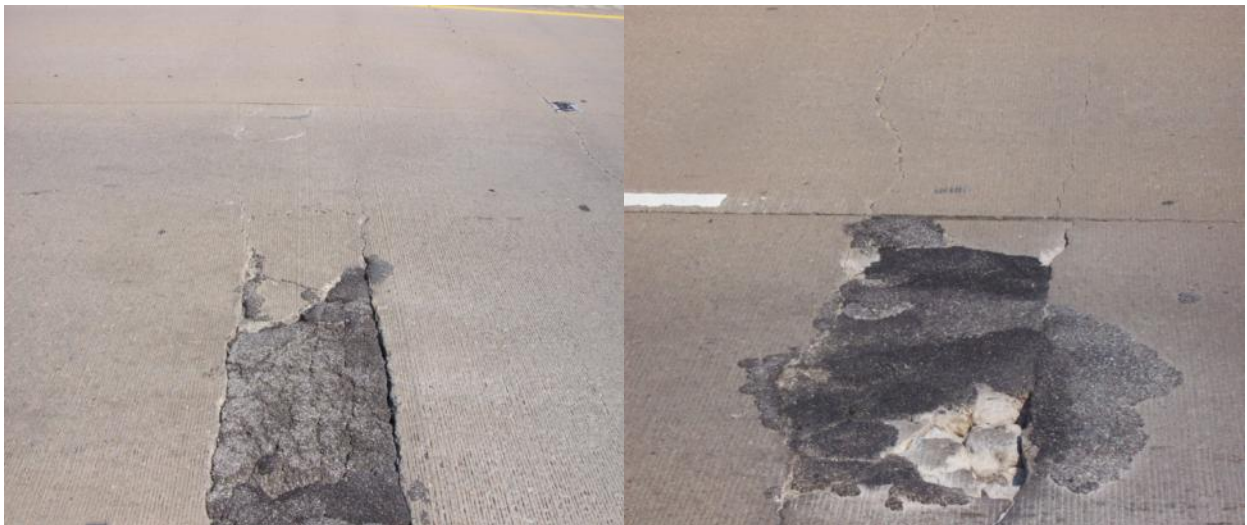
Figure 3.42 – More patches cause by closely spaced transverse cracks
