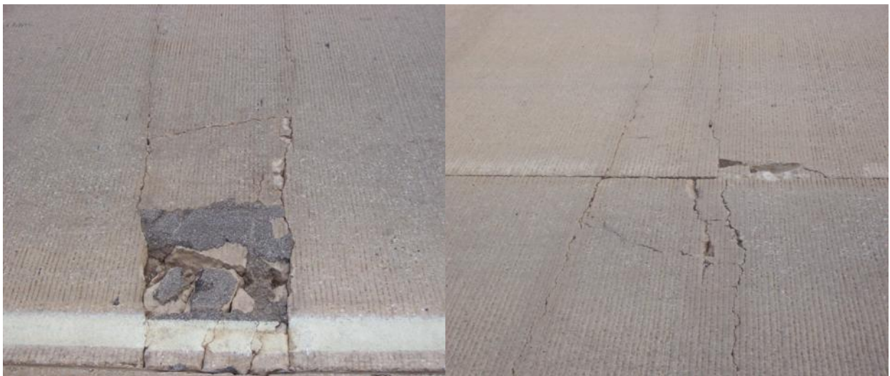
Figure 3.25 – Punch-outs forming between closely spaced transverse cracks
