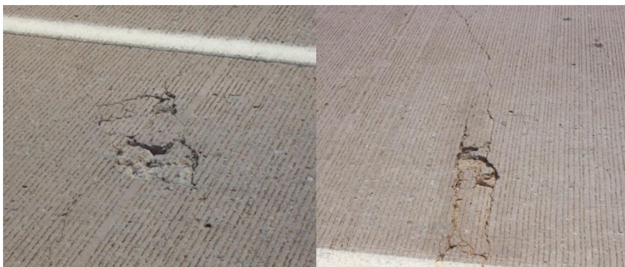
Figure 3.60 – (left) Two closely spaced transverse cracks, (right) Y-crack developing into a punch-out
