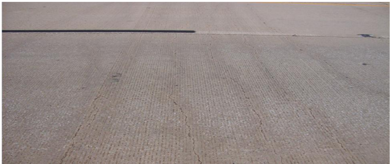
Figure 3.23 – Closely spaced transverse cracks
