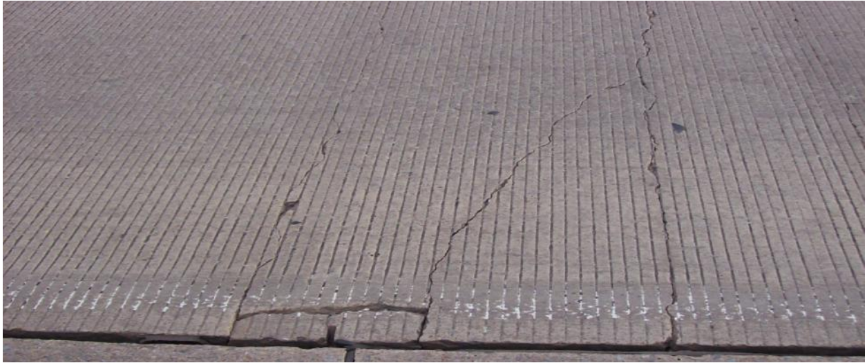
Figure 3.35 – Typical Y-crack for the area
