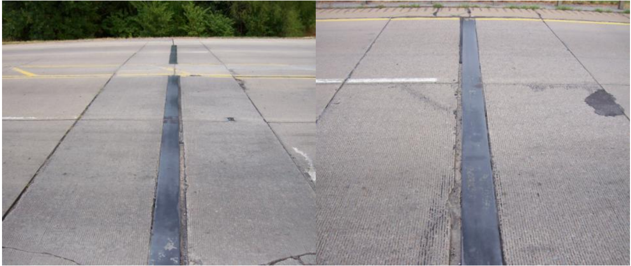
Figure 3.33 – Terminal joints showing signs of spalling
