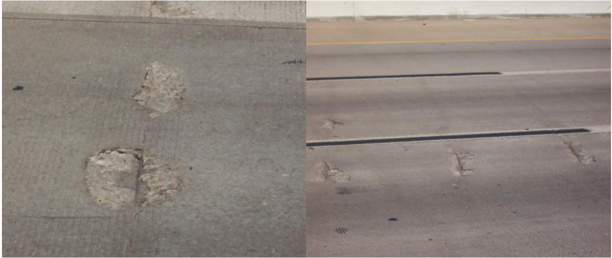
Figure 3.8 – Distresses in ODOT’s region of concern
