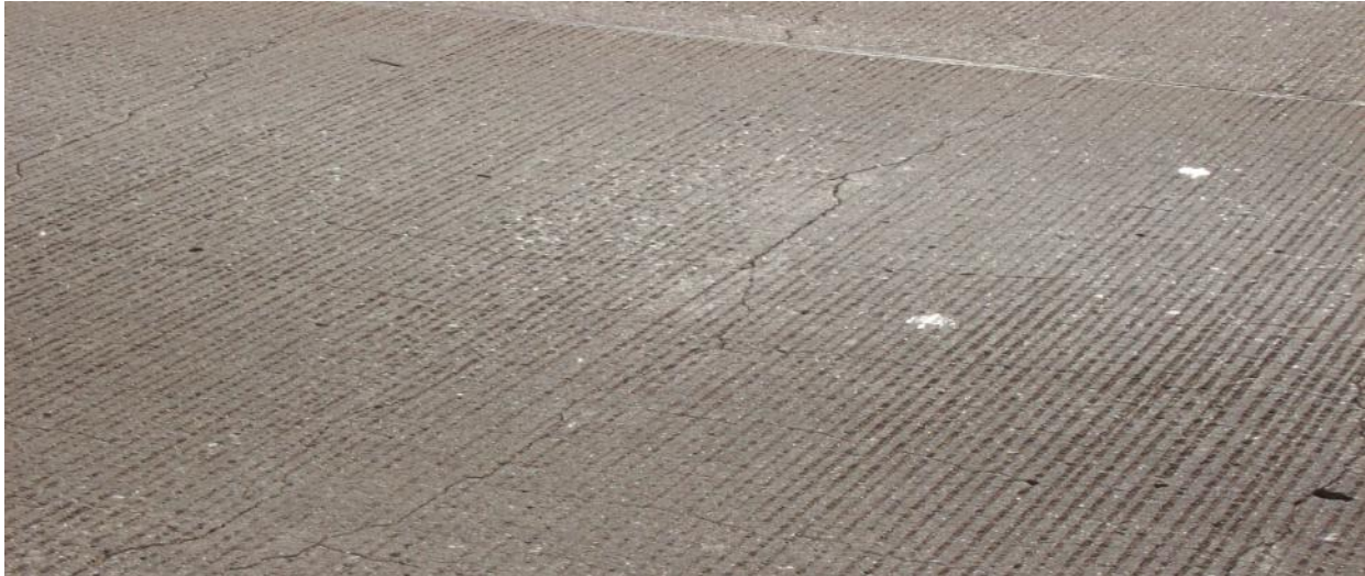
Figure 3.2 – Photo shows transverse cracks with inter-connecting longitudinal cracks.
