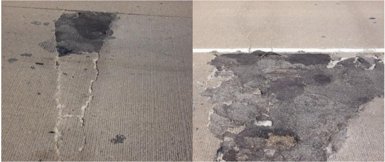
Figure 3.43 – (left) Patch caused by a Y-crack (right) patch with steel protruding through
