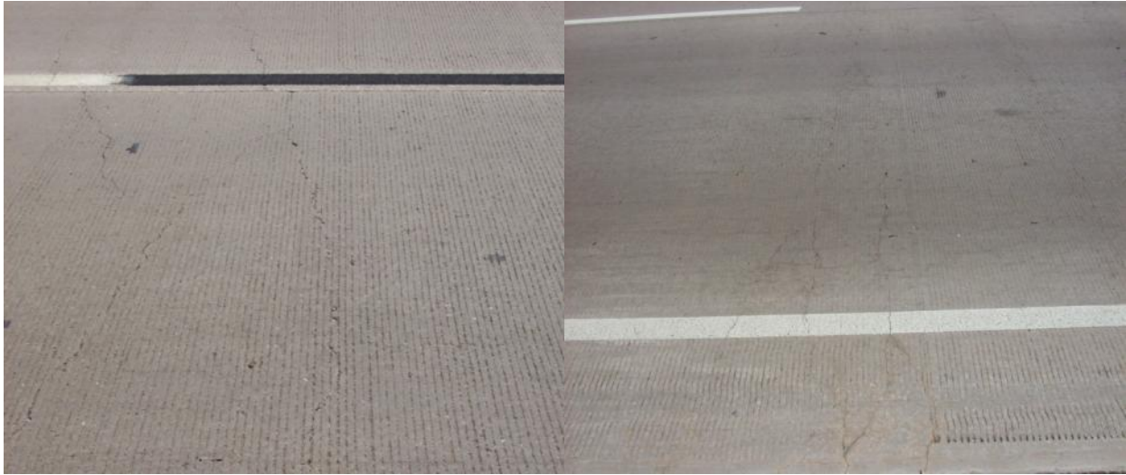
Figure 3.19 – Two different forms of Y-cracking
