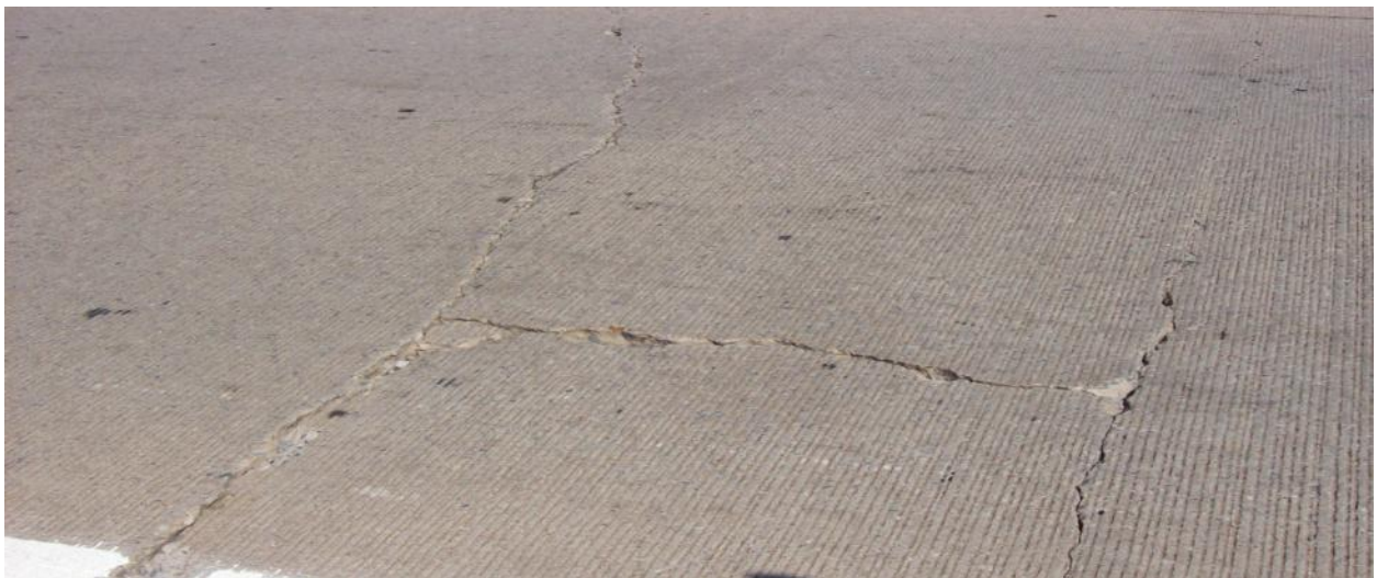
Figure 3.44 – Two transverse cracks intersected by a longitudinal crack
