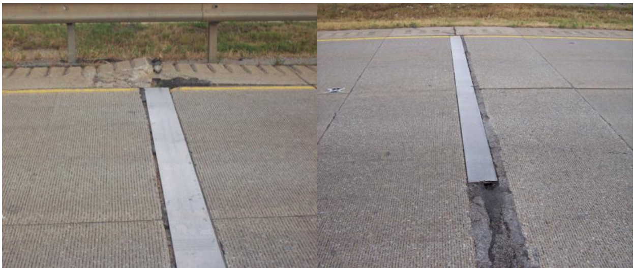
Figure 3.34 – Terminal Joints with different kinds of distress
