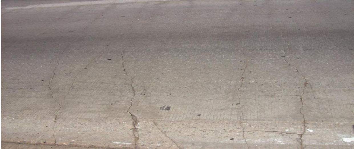
Figure 3.7 – Closely spaced transverse connected by longitudinal cracks
