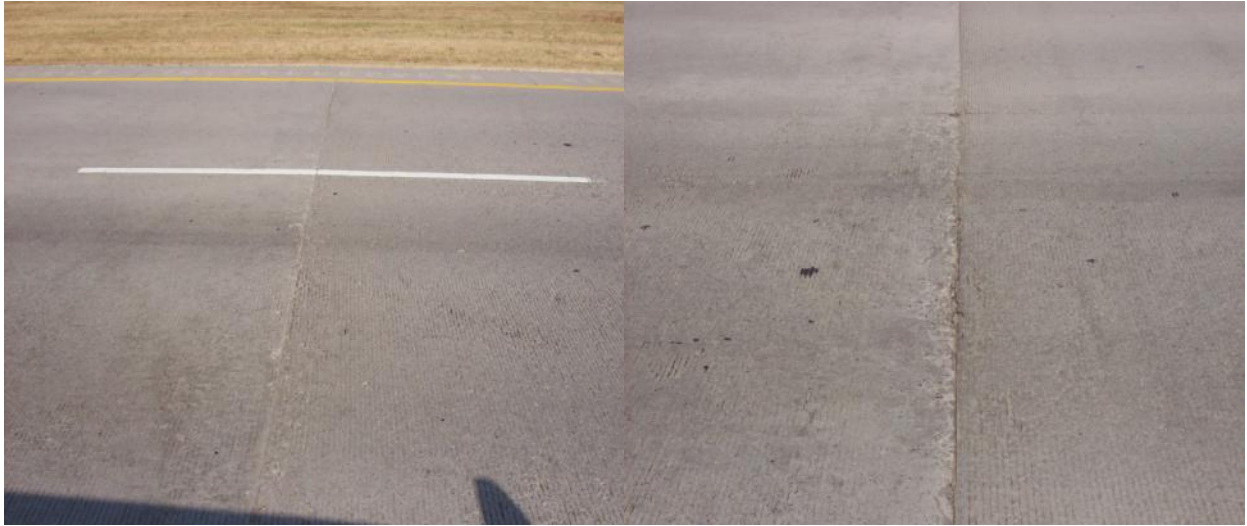
Figure 3.16 – Two construction joints displaying signs of spalling
