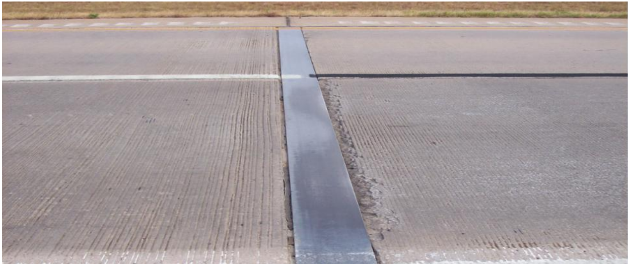
Figure 3.21 – Deteriorated terminal joint at project beginning
