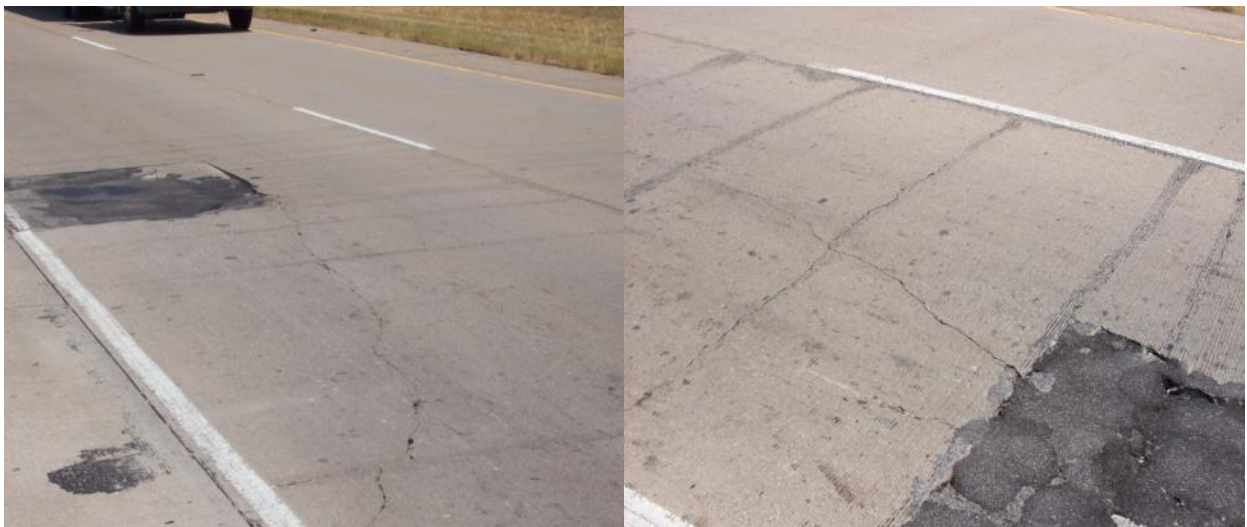
Figure 3.49 – Multiple transverse cracks intersected by a longitudinal crack
