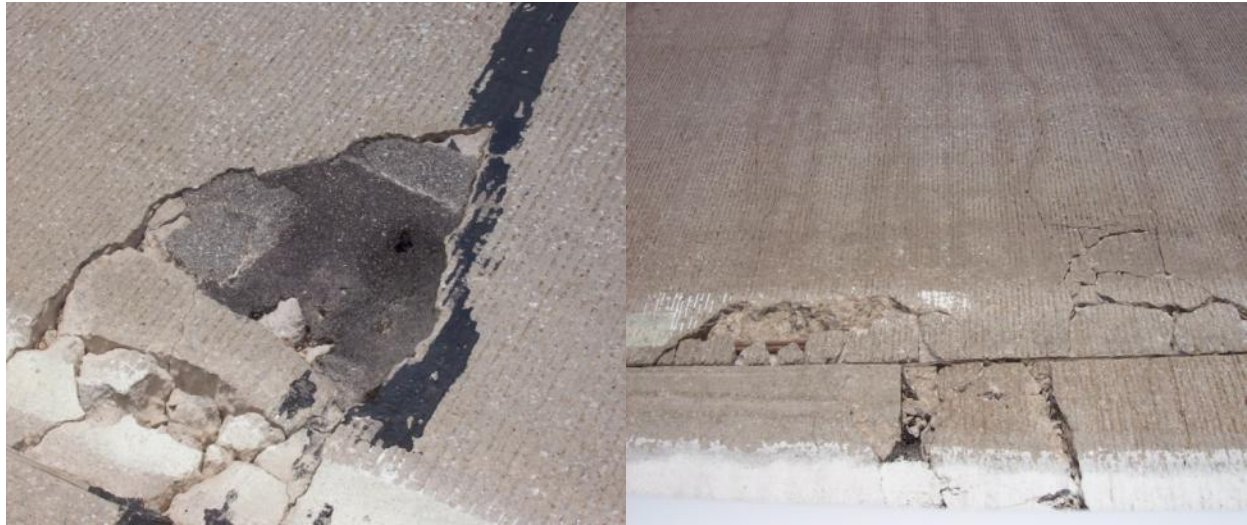
Figure 3.30 – (left) Y-crack breaking up, (right) distress caused by close transverse cracking
