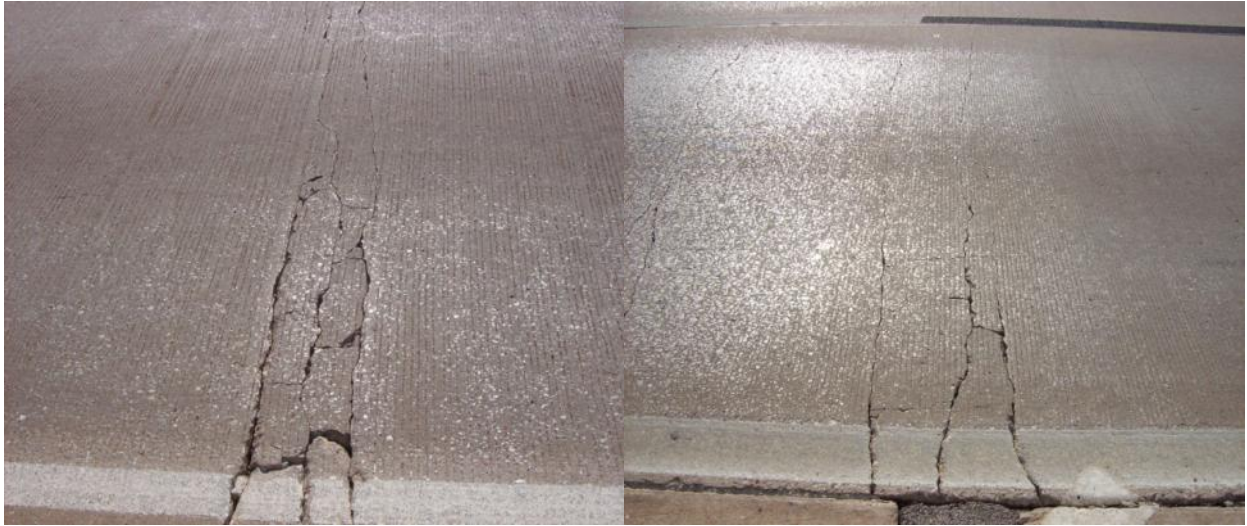
Figure 3.4 – Photo showing closely spaced transverse cracks developing into punch-outs
