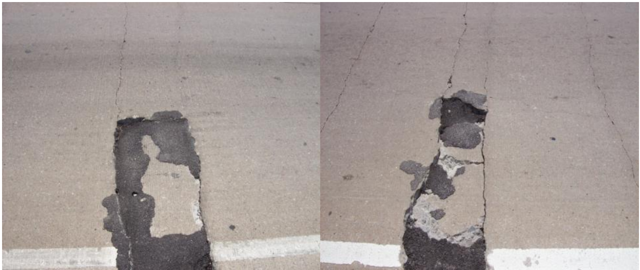
Figure 3.45 – Transverse cracks intersected by longitudinal cracks
