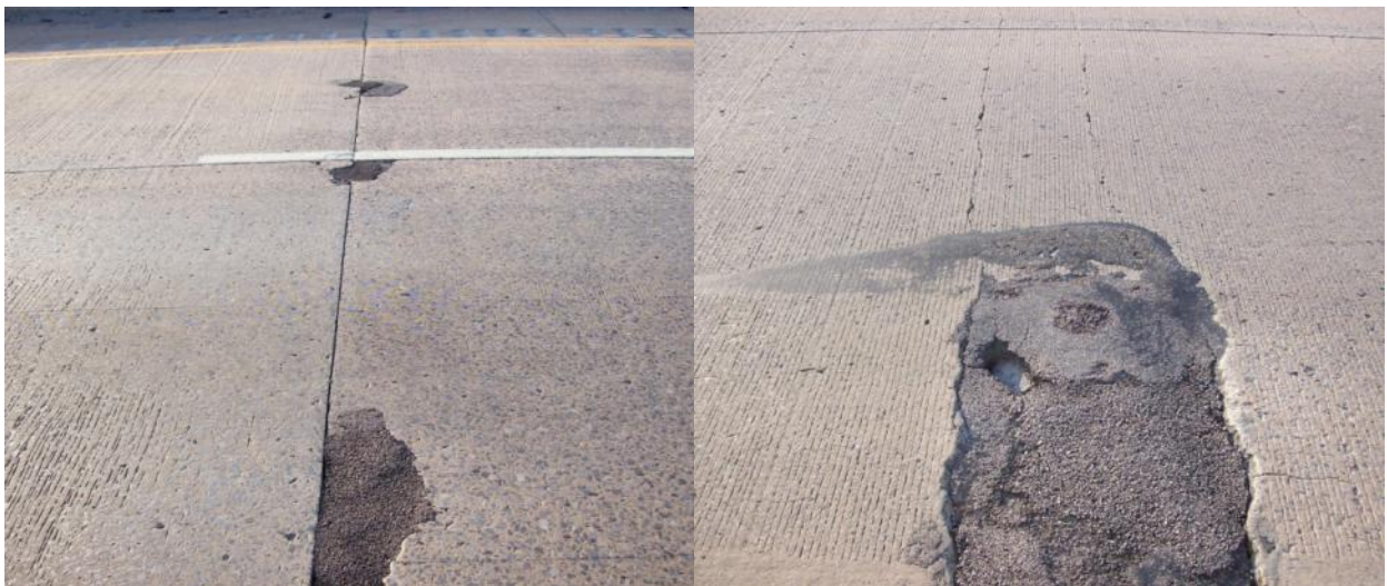
Figure 3.68 – Patches in the south bound lane
