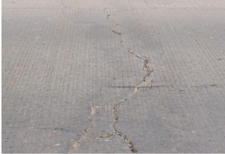
Figure 2.3 - Example of spalling
