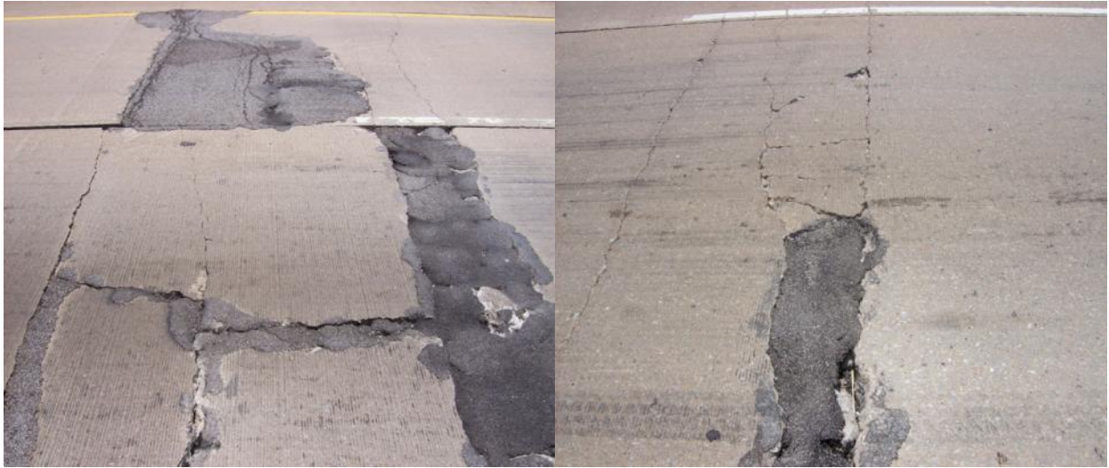
Figure 3.46 – Transverse cracks intersected by longitudinal cracks
