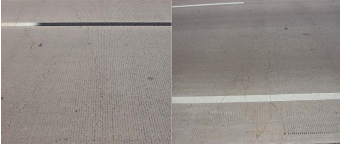
Figure A.19 Two different forms of Y-cracking
