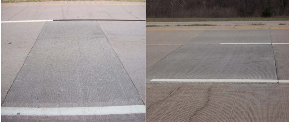
Figure A.74 Patches with longitudinal cracking
