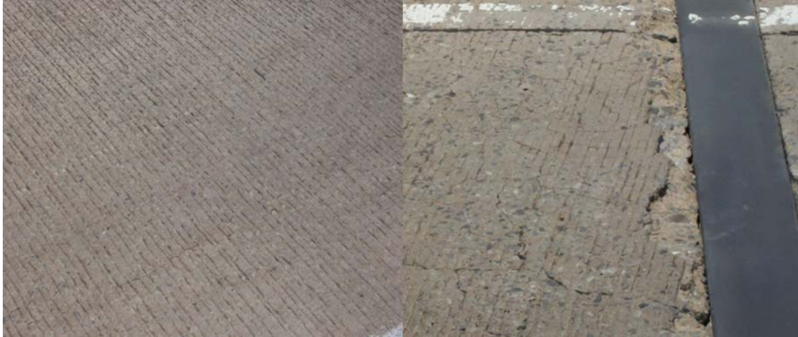
Figure A.65 Close ups showing map-cracking
