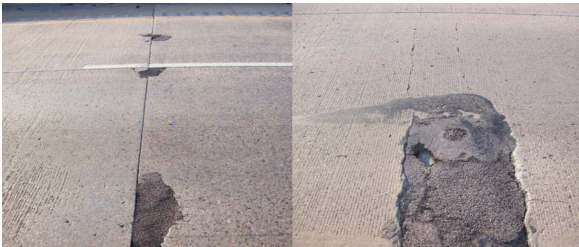
Figure A.68 Patches in the southbound lane
