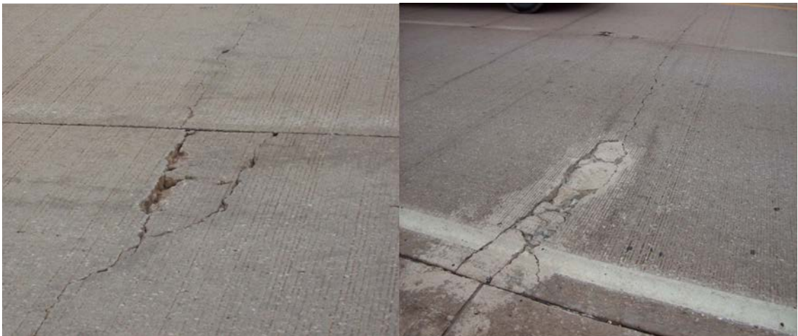
Figure A.77 Punchouts/ patches forming near Y-cracks
