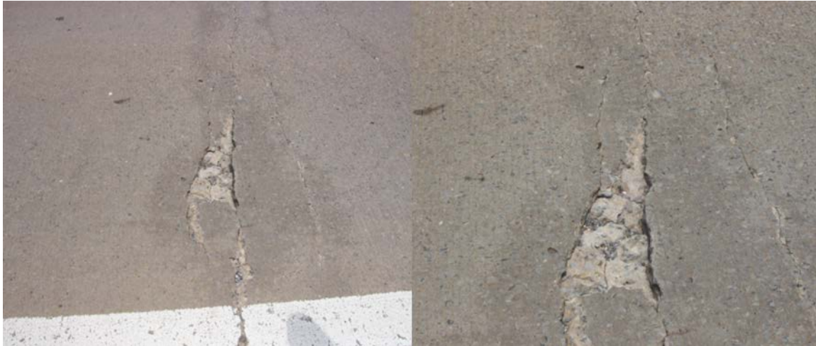
Figure A.62 Y-crack developing into a punch-out
