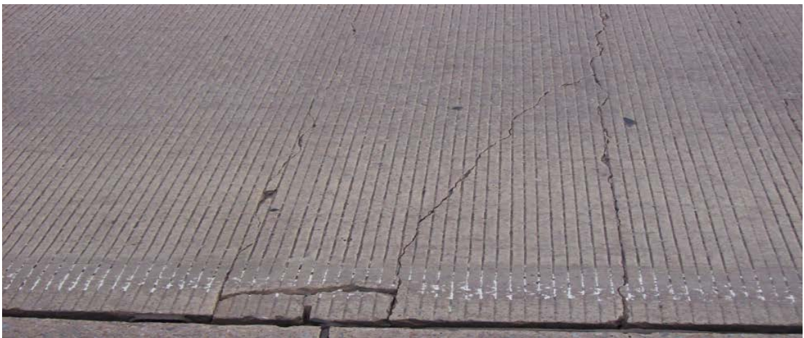
Figure A.35 Typical Y-crack for the area
