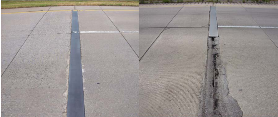
Figure A.37 Terminal joints showing distress
