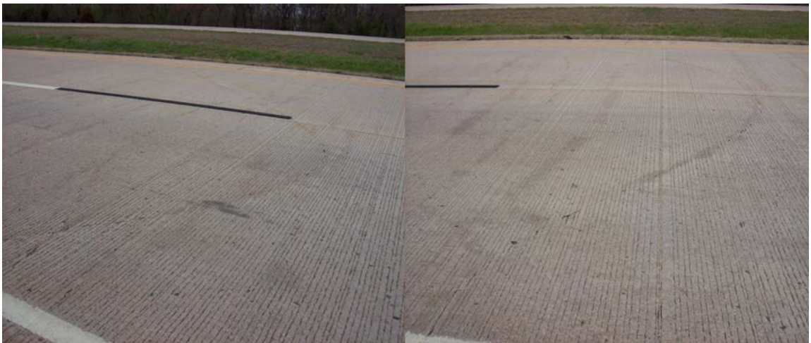
Figure A.90 Circular cracks intersecting transverse cracks
