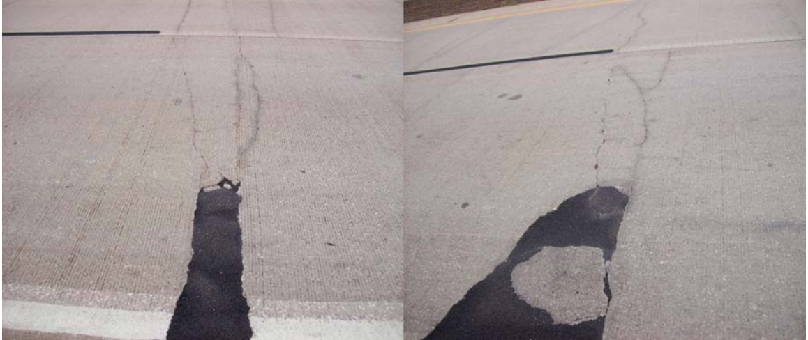
Figure A.76 Punchouts/ patches forming near Y-cracks
