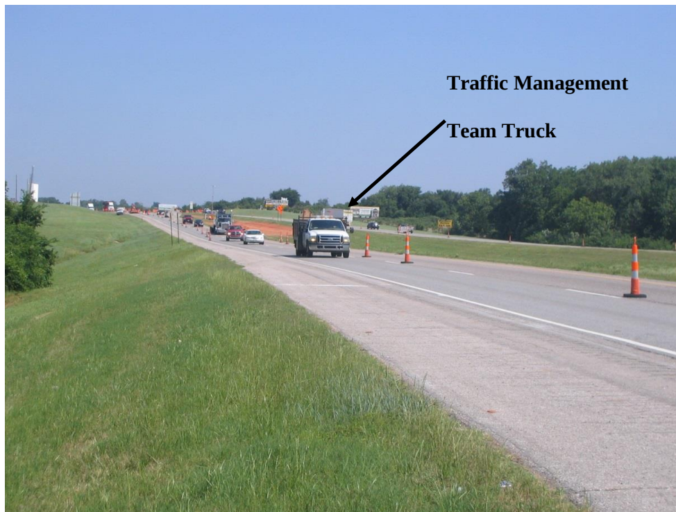
Figure 3-82 Opening of Lane for Traffic
