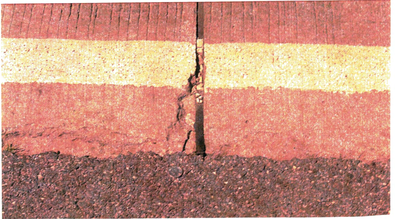
Figure 1 Typical Corner Crack and Spalling at Outside Edge of Slab
