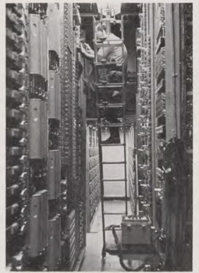
Telephone communications room is the nerve center of building's communication system.
