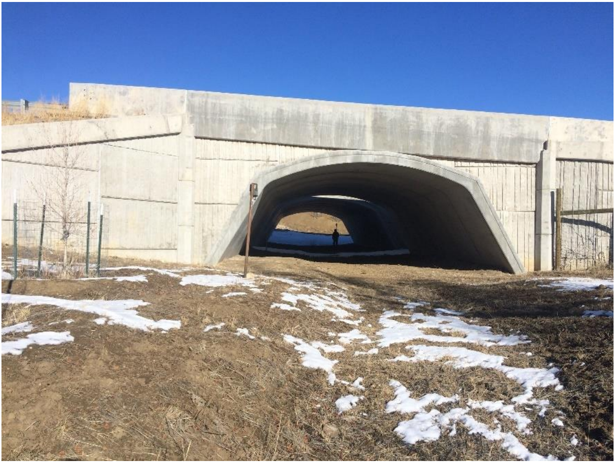
Figure 3. Monitored Wildlife Crossing Structure US 160 MP 97.42. The Monitoring Camera and Post at the South Entrance are in the Foreground. Cameras Faced the Entrances.
