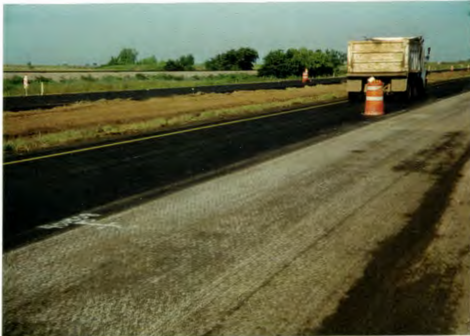
Photo 6. Milled Surface, Section 400508
