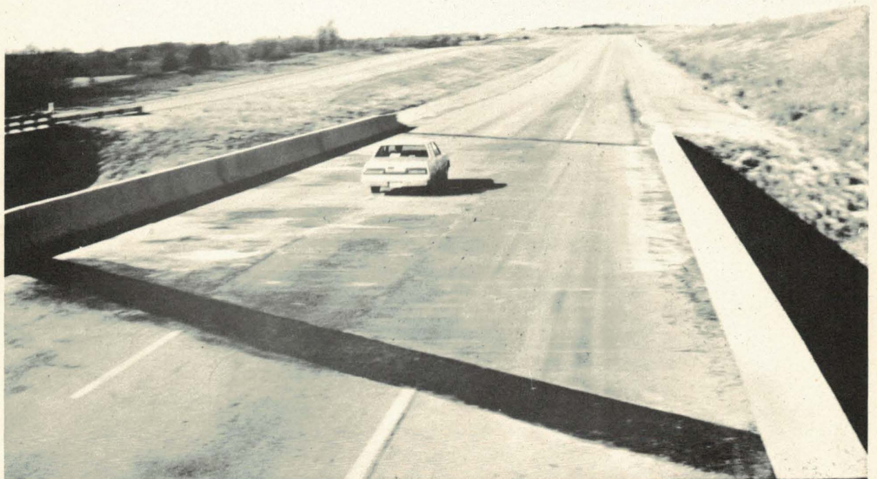
Figure 26. The bridge with its multi-colored patches as it appeared three months after initial construction.
