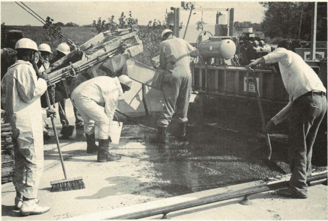
Figure 11. Polymer concrete was discharged onto a tackcoated surface before the paving machine.
