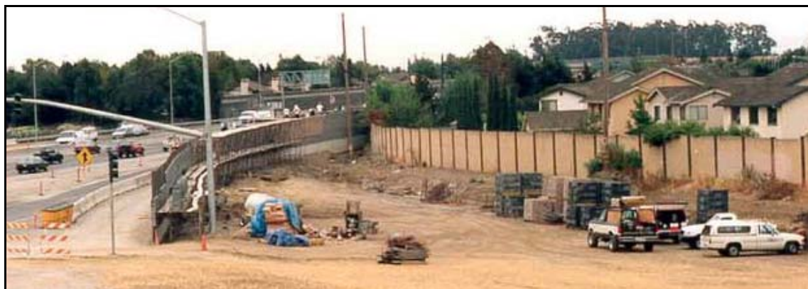
Figure 7.28 Existing noise barrier left in place until replacement noise barrier is constructed (Photo #483)
