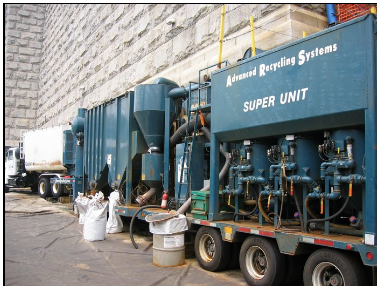
Figure 5.8 Compressors, vacuums, and paint chip collection equipment associated with paint removal operation (Photo #398)
