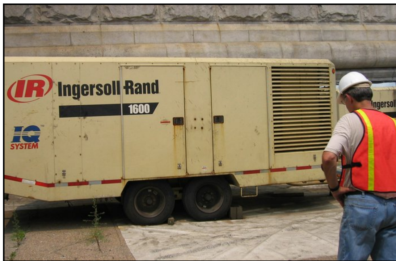
Figure 5.3 Measurement of an individual piece of equipment (Photo #693)
