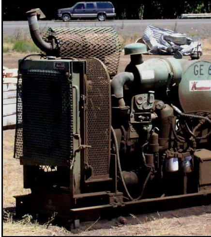
Figure 7.14 Unshielded, non-baffled equipment (Photo #74)
