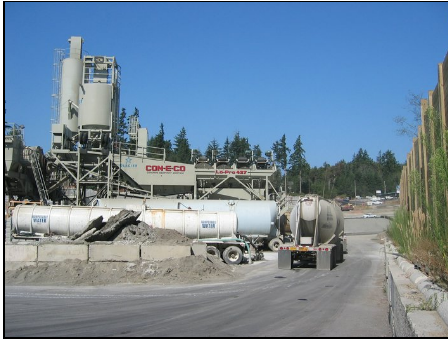
Figure 5.28 Concrete batch plant operation; shown here with temporary noise barrier for community to the right (Photo #322)
