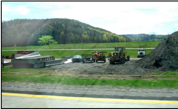
Figure 7.2 Partial shielding of storage area in residential area (Photo #247)
