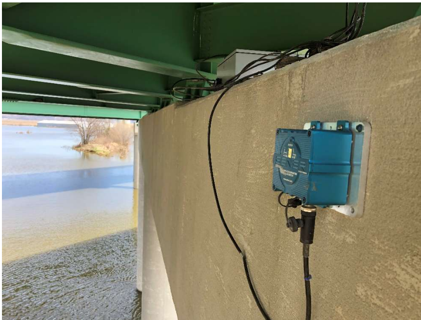
Figure 4. Photograph of SENSR System Deployed on I-29 Bridge
