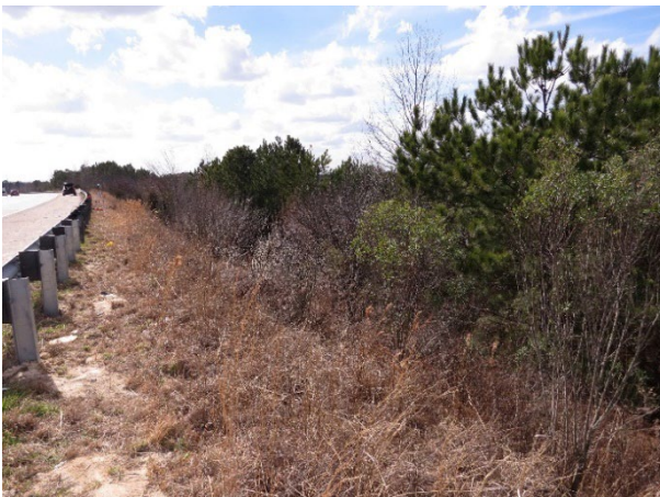
Figure 4. Facing southwest and viewing the shoulder/ embankment drop-off as seen from Event 2
