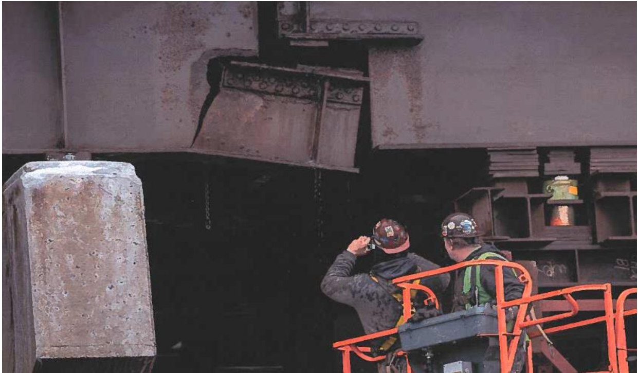
Figure 32b. In this photograph, an expansion joint shelf consisting of equal leg angles bolted to a girder web sustained a crack at a sharp corner due to cantilever action from the adjacent girder, causing crack advancement under repeated cyclic stress due to heavy truck traffic. The failure of the girder web and bending of the lower flange caused a shutdown of the expressway. Temporary supports are shown to keep traffic moving. Crack was discovered on Lake Shore Drive Bridge at Randolph St. in Chicago by electrical crews working on traffic signals. Chicago Tribune photo, dated February 13, 2019.
