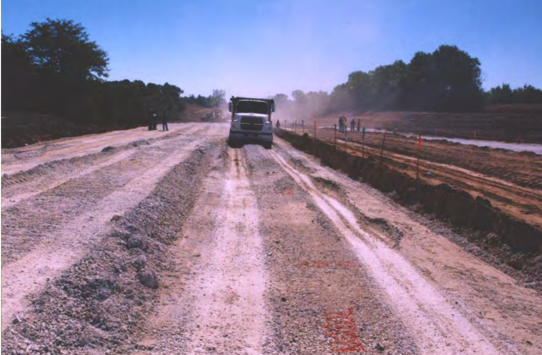
Figure 6. Loading Transition area between Type A (foreground) and Type B (background) CLS CA-6. Note edge effects the right side of the photo corresponding to the left wheel path
